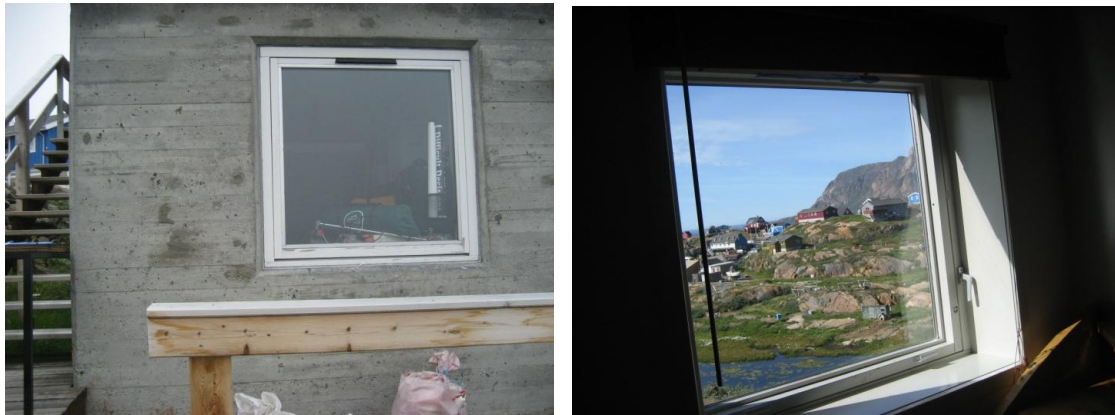
Fig. 13. Windows used in the Blue House
