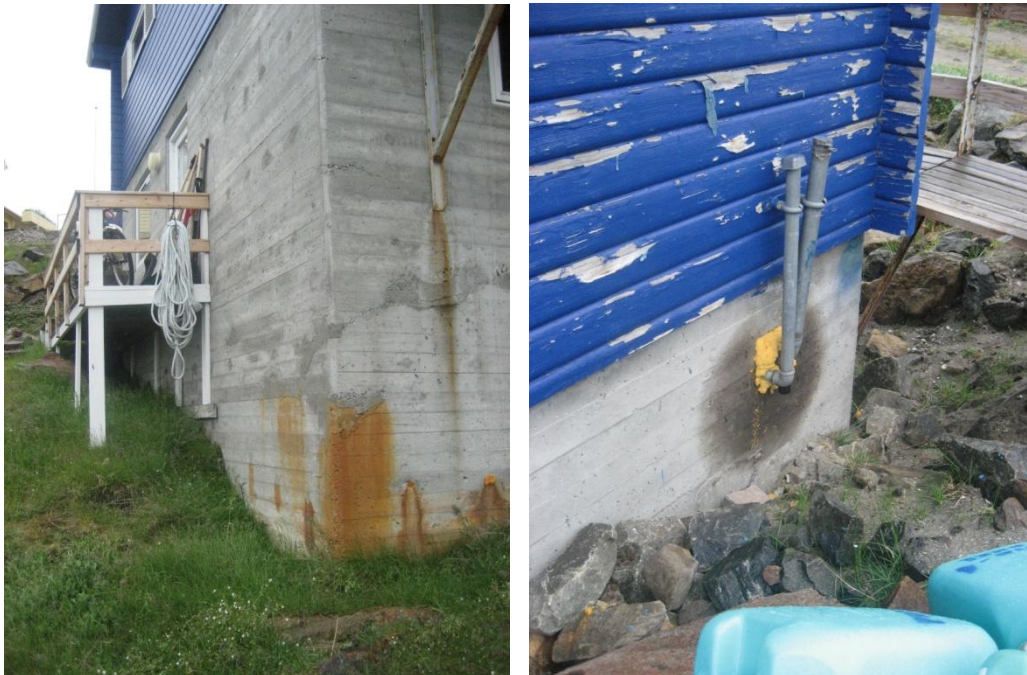
Fig. 17. Cracks in the basement walls (on the left) with water leakages through the foundations and the exterior painting
