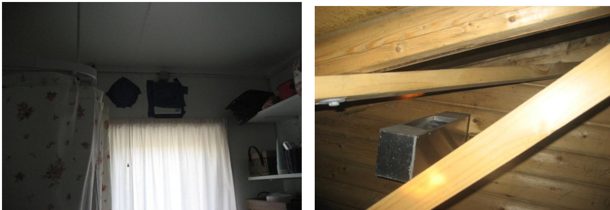
Fig. 16. Mechanical vent in the bathroom and natural ventilation in cold attic
