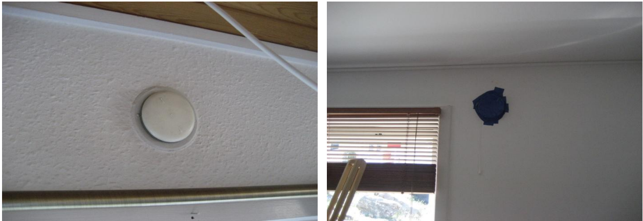
Fig. 15. Natural vents in the first and basement floor
