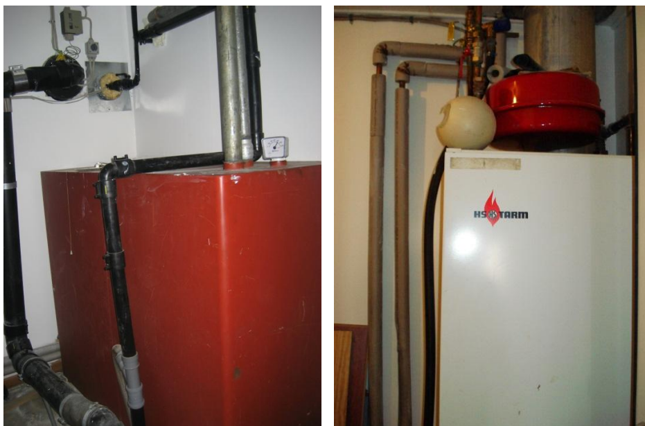
Fig. 14. Oil tank and oil-boiler in the technical room
