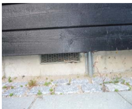
Figur 91 Ventilationsrist i fundament
