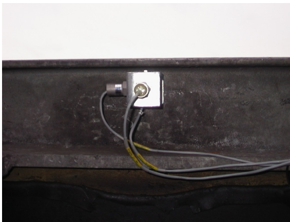
Figure 7: DanControl VC3 accelerometers in the rear of the nacelle
