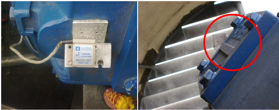
Figure 17: Summit 3-axial accelerometer at generator corner at different viewpoints
