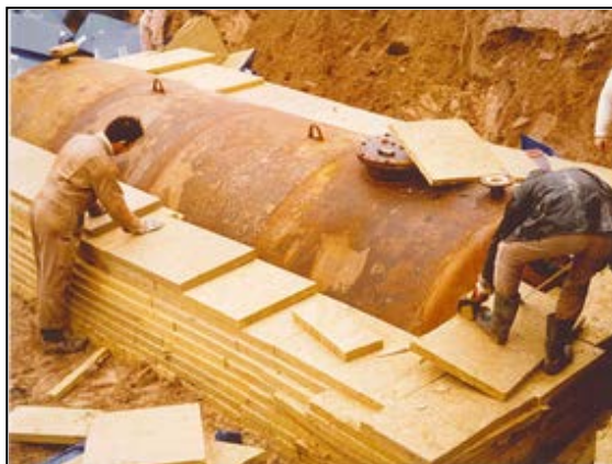
Den store akkumulatortank.
