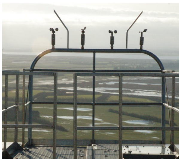
Figure 13.1 Arrangement of nacelle anemometry on the back of the nacelle of modern wind turbines. The instruments are typically mounted on a reasonably solid support structure with lightning protection covering the instruments and with redundant mounting of instruments
