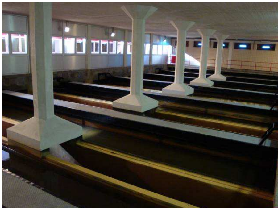
Figure 1.3: First-stage rapid sand filters room at Sjælsø Waterworks, Denmark.
