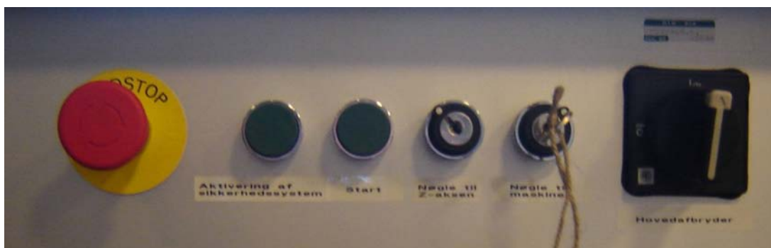
Figure D.2 X-ray system control panel. (Author's photos)
