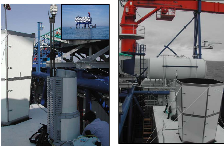
Figure 2.2. Ground-based remote sensing instrumentation on the Horns Rev transformer/platform. To the left: QinetiQ's ZephIR Wind LiDAR. To the right: AQ500 SoDAR.
