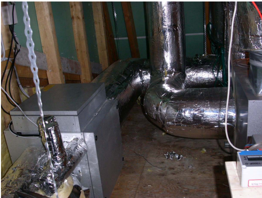
Insulated ducts and the additional heating coil.
