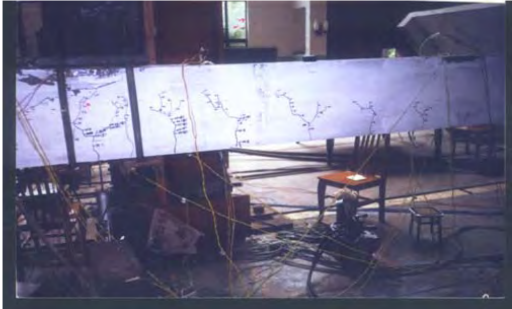
(a) Cracks in span
