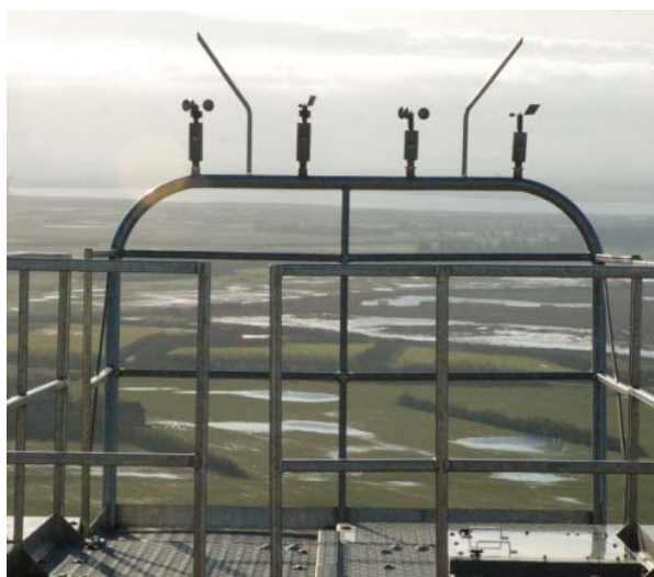
Figure 1 Arrangement of nacelle anemometry on the back of the nacelle of modern wind turbines. The instruments are typically mounted on a reasonably solid support structure with lightning protection covering the instruments and with redundant mounting of instruments
