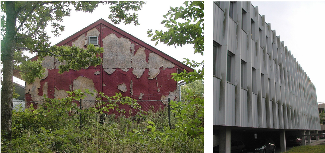
Figure 4.7: Different surface failures. Left: the surface paint is not intact and the underlying material is no longer protected. Right: algae growth at a white aluminium facade. Although the facade is still protected, the surface has failed because the building looks dirty and is in contrast to the image the building owner wants.
