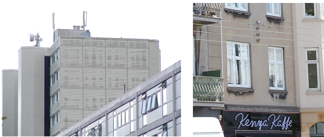
Figure 3.6: Soiling patterns indicate the origin of the dirt. Left: biological growth at exposed moist areas. Right: in polluted areas the rain will wash off some of the particles in unprotected areas. The rain will not clean areas under protective items like sills or coverings. This results in darker areas under protective items.
