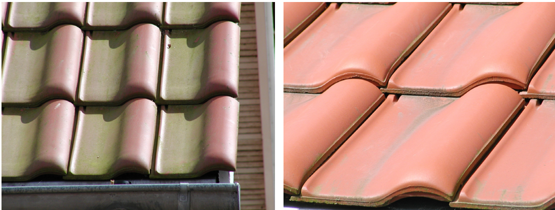
Figure 6.5: Two year old roof with Lotus tiles. Left: north side. Right: south side, notice the same soiling pattern as at the low slope in Figure 5.3 from the field test. The roof was renewed for aesthetic reasons. The old roof of concrete roofing tiles was covered with biological growth and after cleaning it quickly resoiled. Tiles with Lotus Effect were chosen for replacement.
