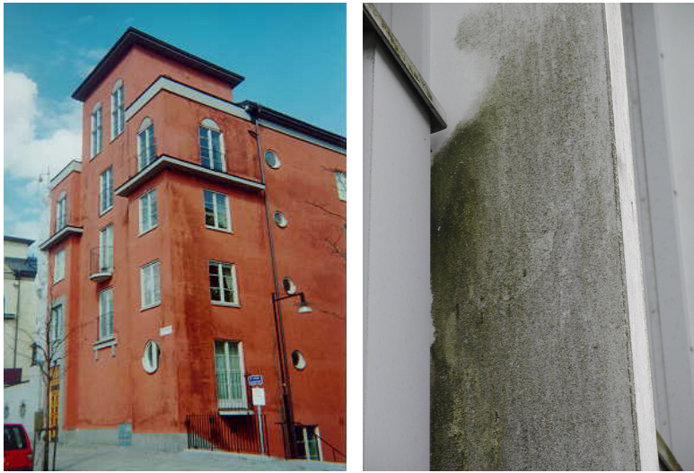
Figure 4.10: Examples of unacceptable soiling. Left: mould growth at a two year old house. Right: Algae growth at aluminium facade, three years after cleaning with brush and water. Both buildings had to be cleaned, despite the risk of higher susceptibility to soiling.
