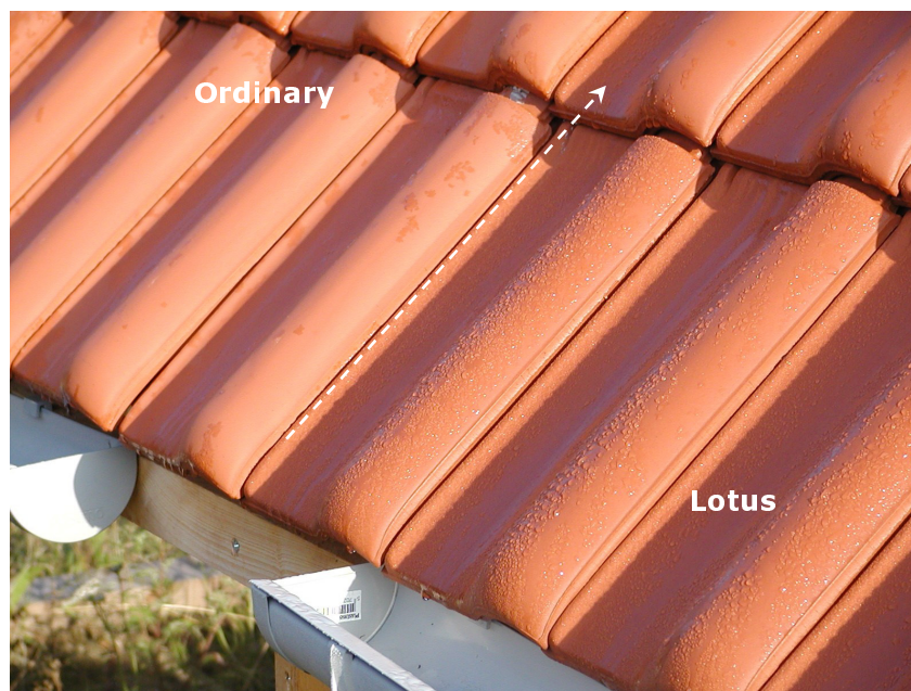
Figure 4.6: Dew at low sloped roofing tiles, left: ordinary tiles. Right: tiles with surface treatment. The dew is not transported from the treated surface into the material; the surface stays wet, while the surface at the ordinary tiles is drying fast. The used surface treatment did not prevent water uptake and was therefore not hydrophobic (see Section 6.1.3.1). However, in some situations, like this, water formed droplets beads, as if the contact angle was > 90^\circ .
