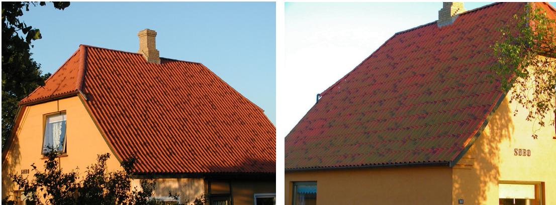
Figure 3.2: Eternite (fibre cement) roof fabricated with “pre-soiling” patterns. The patterns give the surface more life but are different from the natural soiling pattern. At the northern side of the roof (to the right) algae growth has resulted in a greenish discolouration of the roof.
