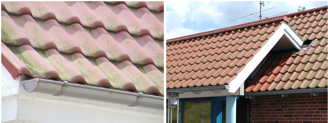
Figure 6.15: Tiles with Lotus Effect. Even at relatively high slopes, approximately 45^\circ the regular parts of the tiles are soiled by biological growth after two years of exposure. Left: north side of roof near a pig farm. Right: north side of roof, notice that the protected tiles under the eaves are clean. From the same house as Figure 6.5 (located close to a bay).
