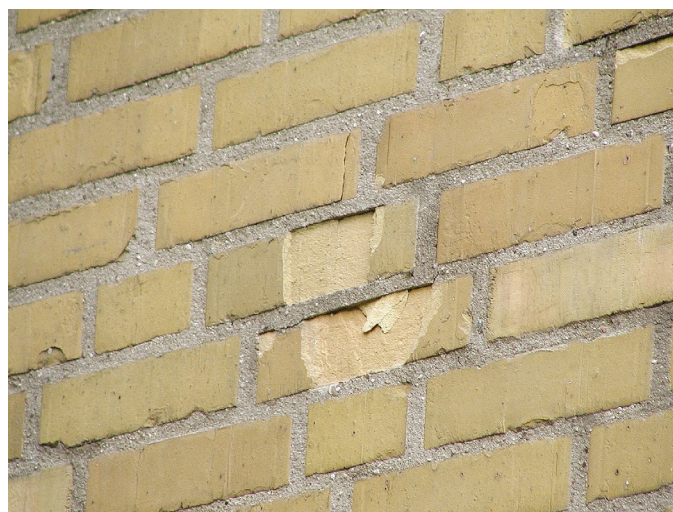
Figure 4.1: Scaling of bricks due to frost damage. Some of the bricks in this detached wall are not frost resistant; 0.5 cm thick layers scale off the brick.
