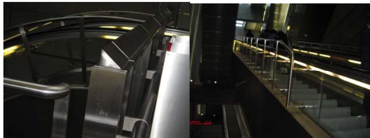
Figure 11. Pictures showing the additional devices installed to enhance the safety inside stations. To the flat veranda (left) designers added a triangular parallelepiped solid piece to prevent people from sitting in the veranda and falling into the three- storey high spaces conceived to provide air and light inside the station. To the escalators, designers added an additional rigid hand rail (right) to prevent people from playing and falling over the moving handrail of the electric escalator.
