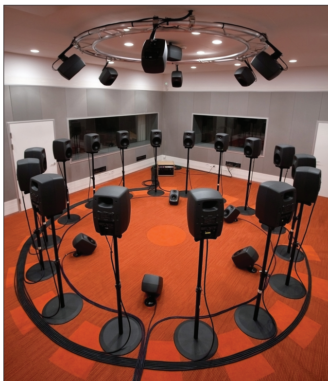
Figure 1. The virtual sound environment (VSE) system installed in one of Oticon's sound studios.
