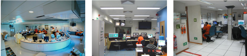
Figure 2: Control rooms with consoles positioned near each other, with the supervisor's work position near the operation consoles and the automation team work position inside the operation environment
