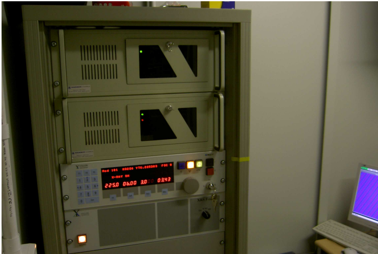
Figure 5-9 Cabinet from which the x-ray is controlled. This is where the kV and the mA for the x-ray are set. These parameters need to be adjusted considering the geometry and the alloy being cast.
