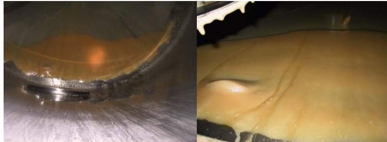
Figure A.4. Salt sticking to tank bottom. Left hand picture was shot from the top of the tank, while the right hand picture was taken through a man hole.
