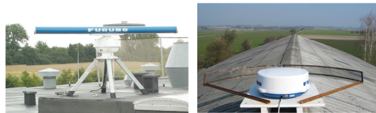
Figure 2 Example of LAWR installations. The LAWR on the left is a standard LAWR. The one on the right is a City-LAWR. Besides the antenna unit on the image there is a small cabinet with two PC's and the radar control unit.
