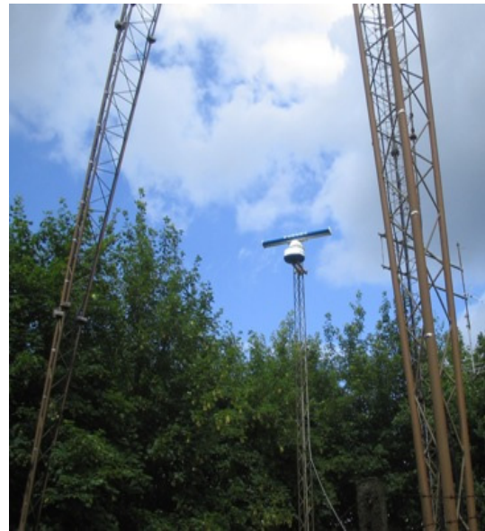
Figure 5.27 Picture of the Aarhus LAW installed underneath a lattice mast surrounded by trees which have grown high enough to cause shielding
