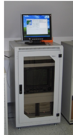
Figure 5.5 Example of the equipment at ground. The radar monitor, 2 PC's, screen and keyboard are all fitted into a rack.
