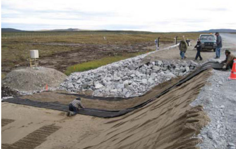
Figure 2.18 Installation of the geocomposite into the shoulder of the runway at Tasiujaq Airport (Doré et. al, 2007)
