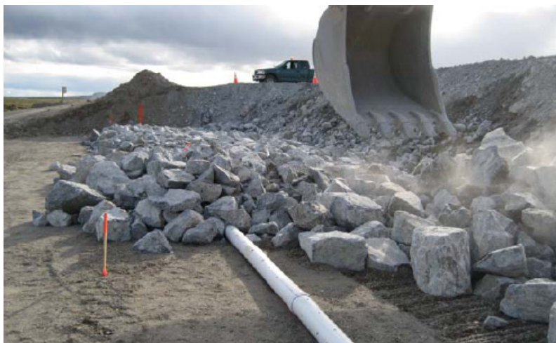
Figure 2.4 Construction of the air convection embankment along the runway at Tasiujaq Airport. The intake ventilation pipe, which will allow cold air to penetrate the embankment, is seen in the bottom of the picture (Doré et. al, 2007)
