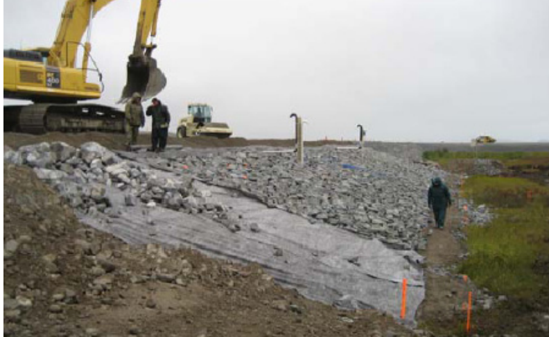
Figure 2.5 Installation of geotextile in the upper part of the air convection embankment (Doré et. al, 2007)
