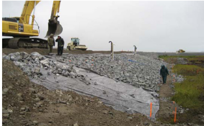
Figure 4. Installation of geotextile in the upper part of the air convection embankment (Doré et al., 2007)
