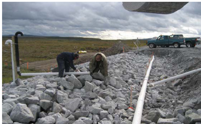
Figure 3. Installation of the ventilation system in the air convection embankment (Doré et al., 2007)
