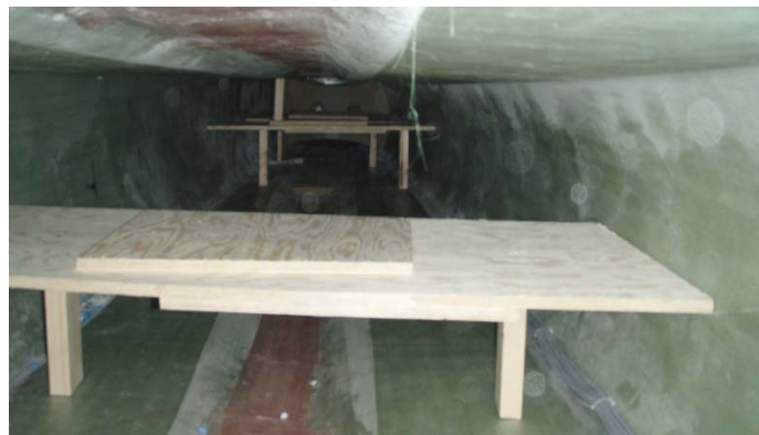
Figure 19. Additional longitudinal bulkheads, to prevent buckling failure at height load. The legs under the plates were used to secure the plate position.
