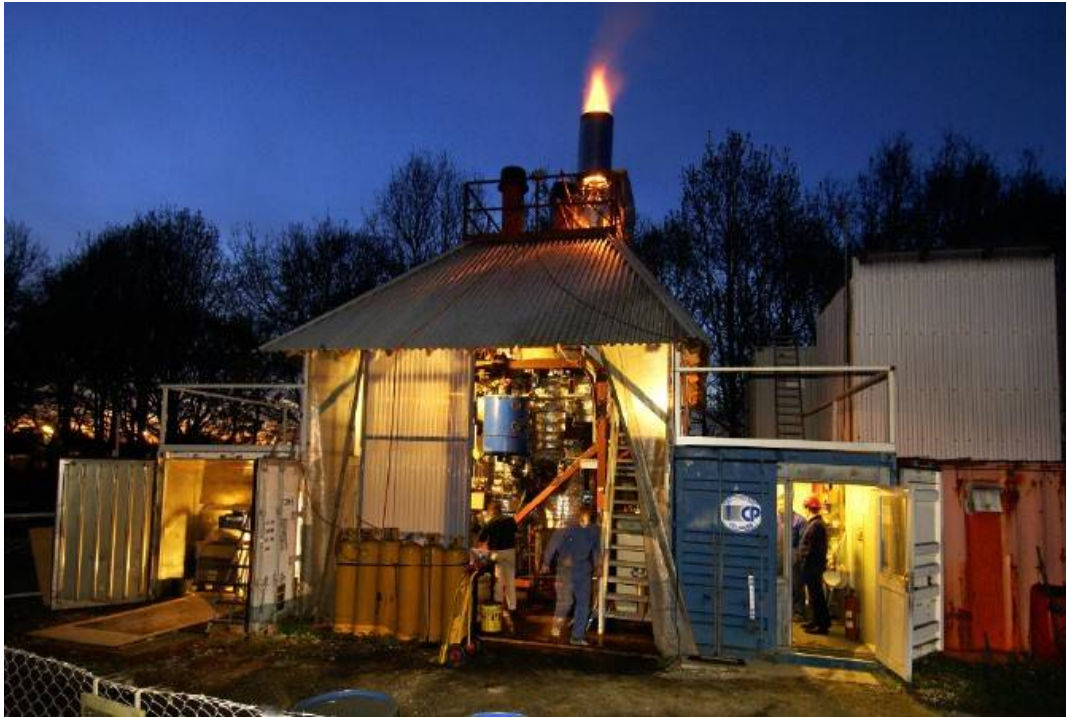
Figure 2.13 500 kW th LT-CFB test plant at DTU
