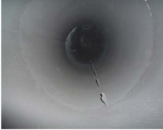
Figure 4.14 Inside view of the cooler after operation
