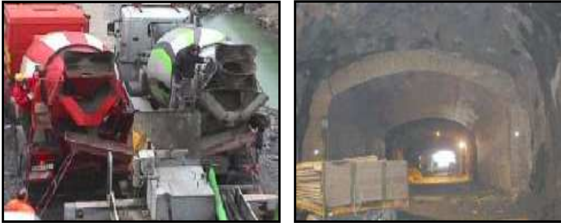
Figure 2.2 The final tunnel lining for the Södra Länken project. The concrete arches were cast with SCC due to the complexity of the structure. To the left the arrangement for continuous discharge, and to the right a view of the south arch (Österberg 2002).
