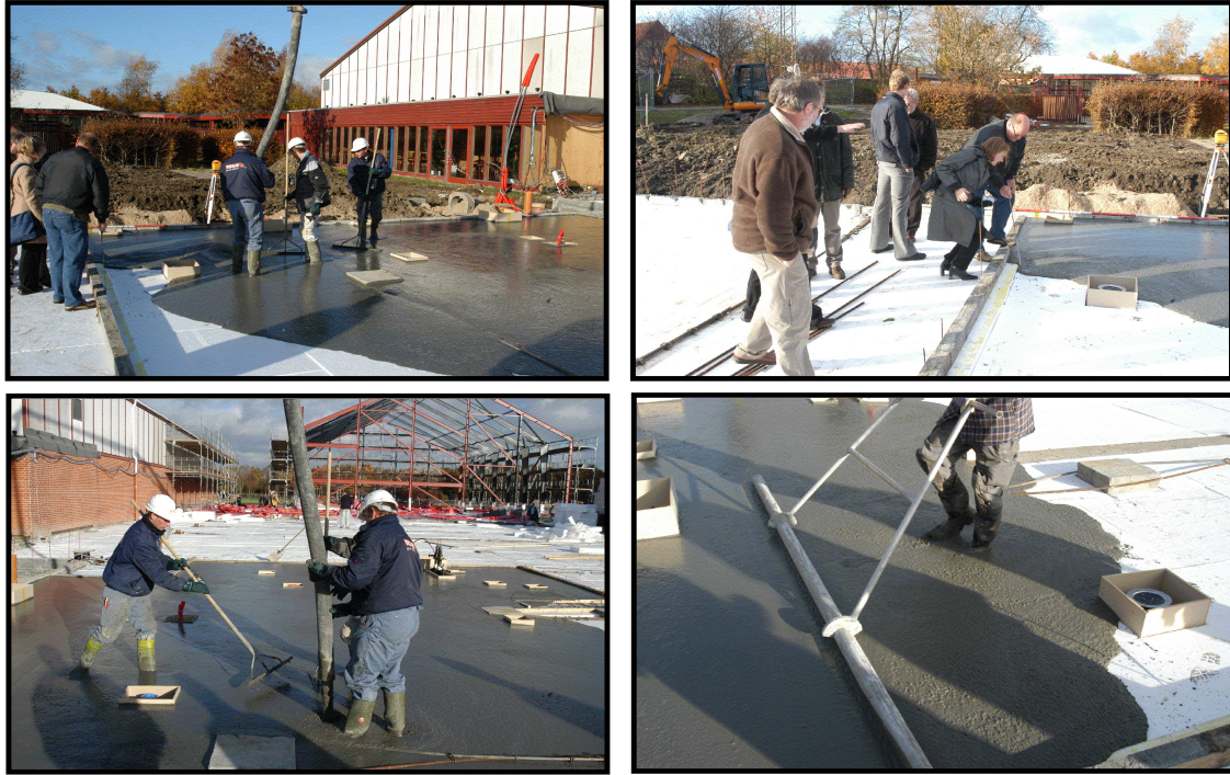
Figure 2.1 An example of a simple horizontal SCC application, in this case an in-situ floor. Drainpipes are typically used to level the surface (Wallin 2003).
