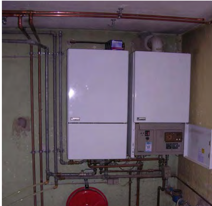
Fig. 6–6 The non condensing natural gas boiler (right) and the hot water tank (left).
