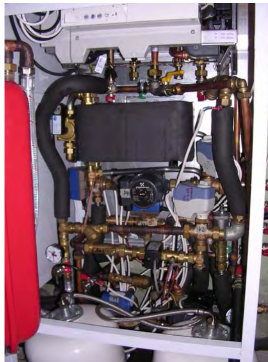
Fig. 6–11 Hydraulic unit inside the technical cabinet in the demonstration system; the big black box is the insulated domestic hot water heat exchanger, below the main pump P4 can be seen.
