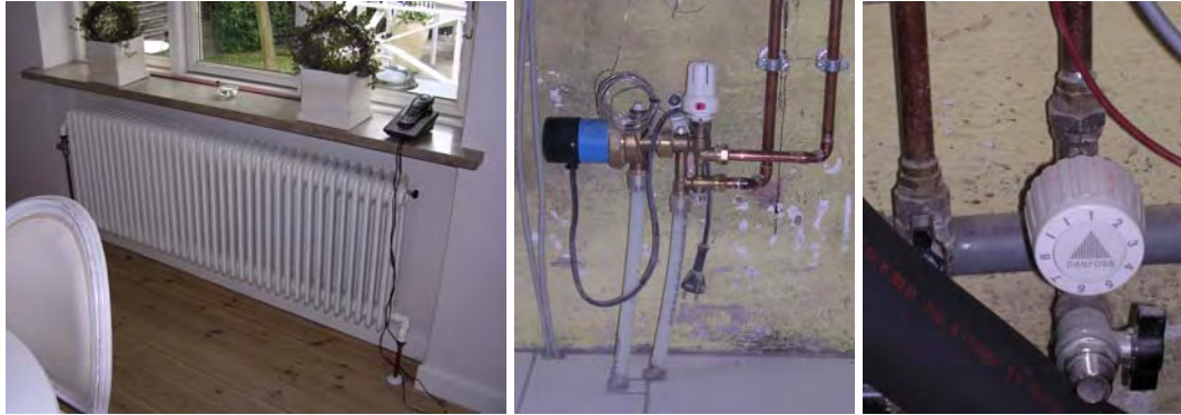
Fig. 6–2 Cast iron radiator in the dining room (left), the pump with integrated mixing valve for the bedroom in the basement (middle) and the return flow control thermostat valve for the floor heating in the bathroom in the basement (right).
