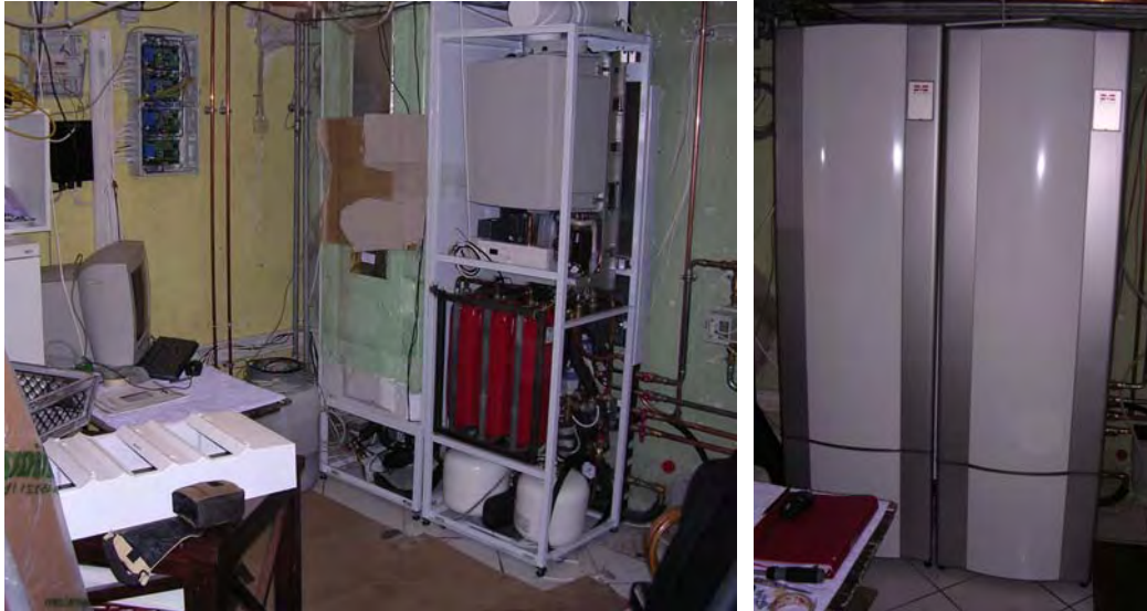
Fig. 6–12 Installation after set in operation on 22/6-2006 (left) and after closing the cabinets with the cover plates (right).
