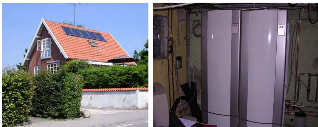
Fig. 6–8 Demonstration house with the collectors mounted on the roof (left) and the installed solar tank unit and the technical unit in the basement (right).
