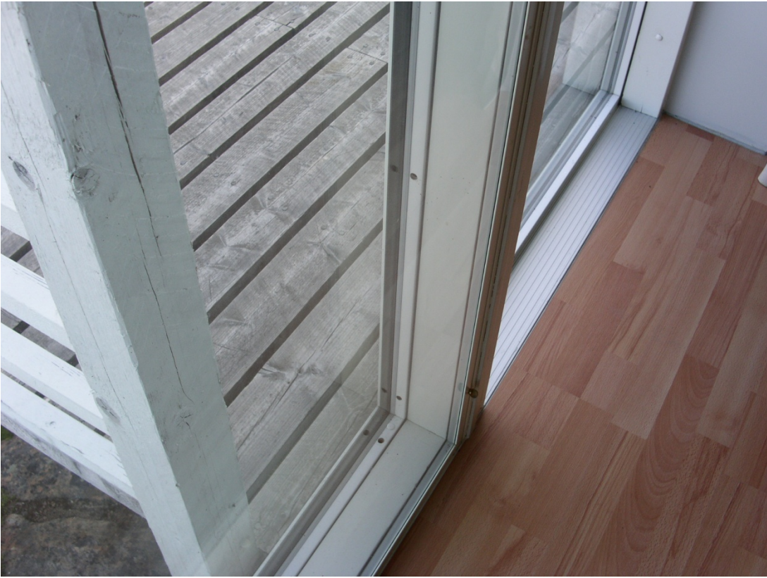
Figure 34 Holes in windows to prevent freezing in winter
