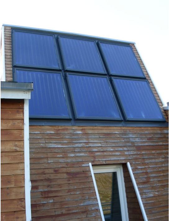
Figure 30 Solar collectors and South facade
