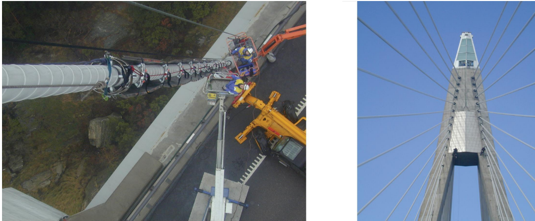
Figure 4: Photos of the PETD system installed on the Uddevalla Bridge after Kuhn (2006).
