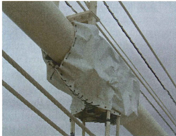
Figure 5: Cable band cover installed on Hakucho Bridge after Numata and Kitada (2008).
