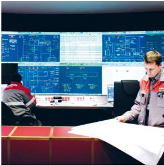
Source: Dong Energy
