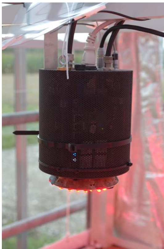
Figure 1 Photo of a LED lamp mounted in the greenhouse
