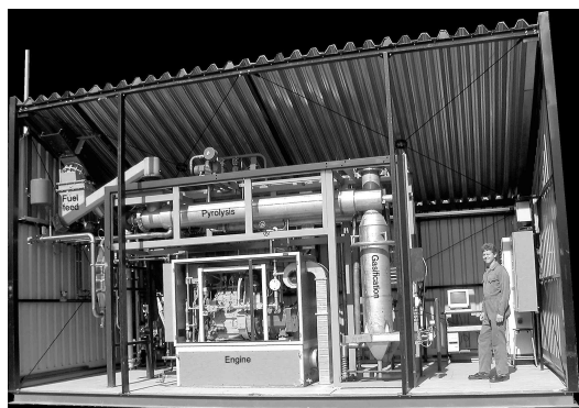
Figure 3: 80-kW pilot plant at DTU
