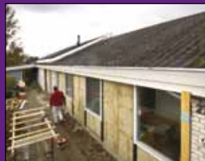
Insulation of existing exterior walls under construction in typical home from the 70's. Photo: Rockwool
