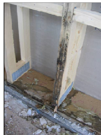
FIG 4. Microbial growth on sole plate and studs, caused by inward leakage of water. Picture from the outside.
