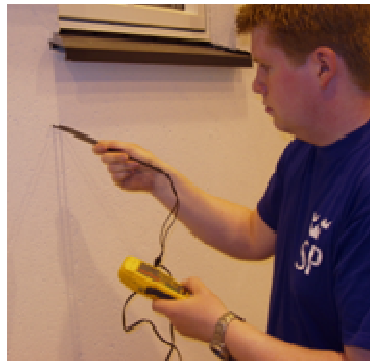
FIG 9. Inserting insulated probes in an upward direction through the holes and through the external insulation.
