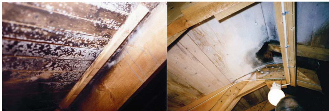
FIG. 1: Example of moisture damaged attics.
