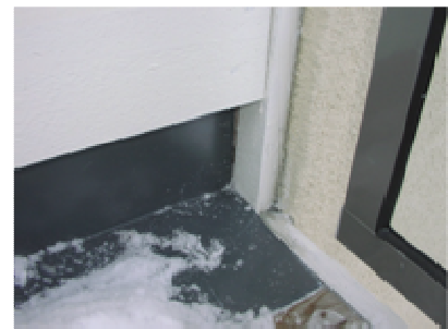
FIG 13. Leaks around the edge of a balcony.
