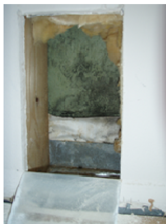
FIG 3. Microbial growth on the outer gypsum board, caused by water leaking in through a defective connection. Picture from the inside.
