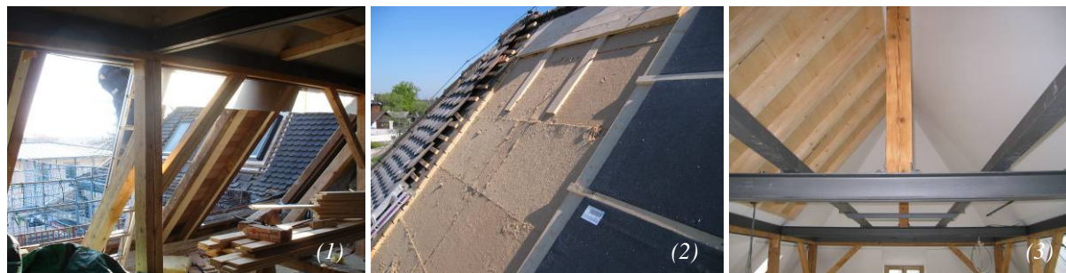
Fig. 4: insulation over the rafters – open roof structure (1), wood fiber insulation boards and vacuum insulation panels (2), completed roof structure (3, on the left: fields of insulation over the rafters)
