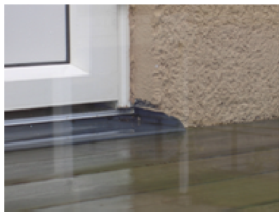
FIG 11. A poor connection to a patio door.
