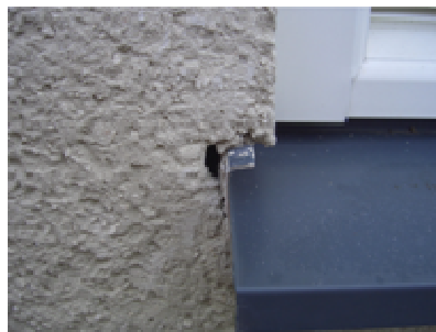
FIG 12. A poor connection around a window
