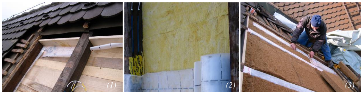
Fig. 3: Variation 2 under construction – open roof with boarding (1), vapour barrier over rafters (2), installation of hemp insulation (3)
