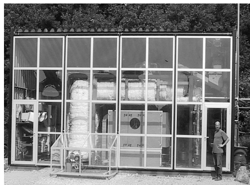
Figure 1. VIKING two-stage gasifier at DTU
