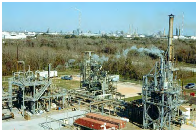
Haldor Topsøe A/S TIGAS process demonstration unit in Houston Texas.
