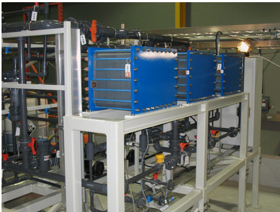
Figure 4 15kW vanadium battery for Risø during factory test
