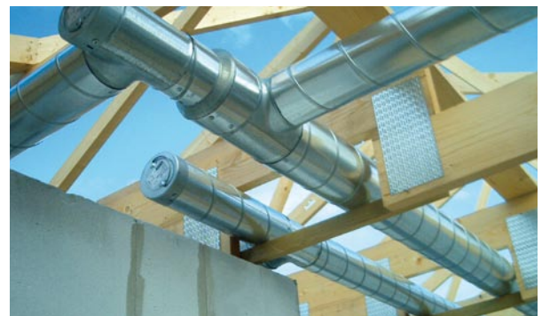
Figure 11: Extending the depth of the rafters in a low-energy house allows ventilation ducts to be installed in a warm ceiling space instead of in the cold attic.
