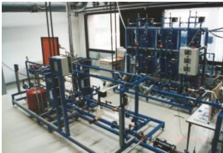
Figure 2.4: Experimental setup at the Danish Technological Institute. The heating system corresponds in capacity to 20 apartments, consisting of three water tanks, heat exchangers, valves, pumps and pipes as well as data acquisition equipment.
