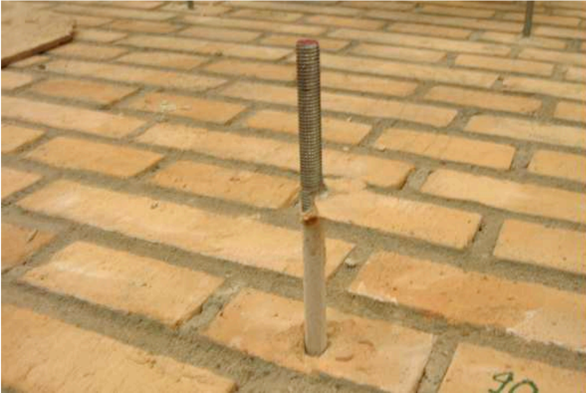
Figure A.51: The failure mode observed
