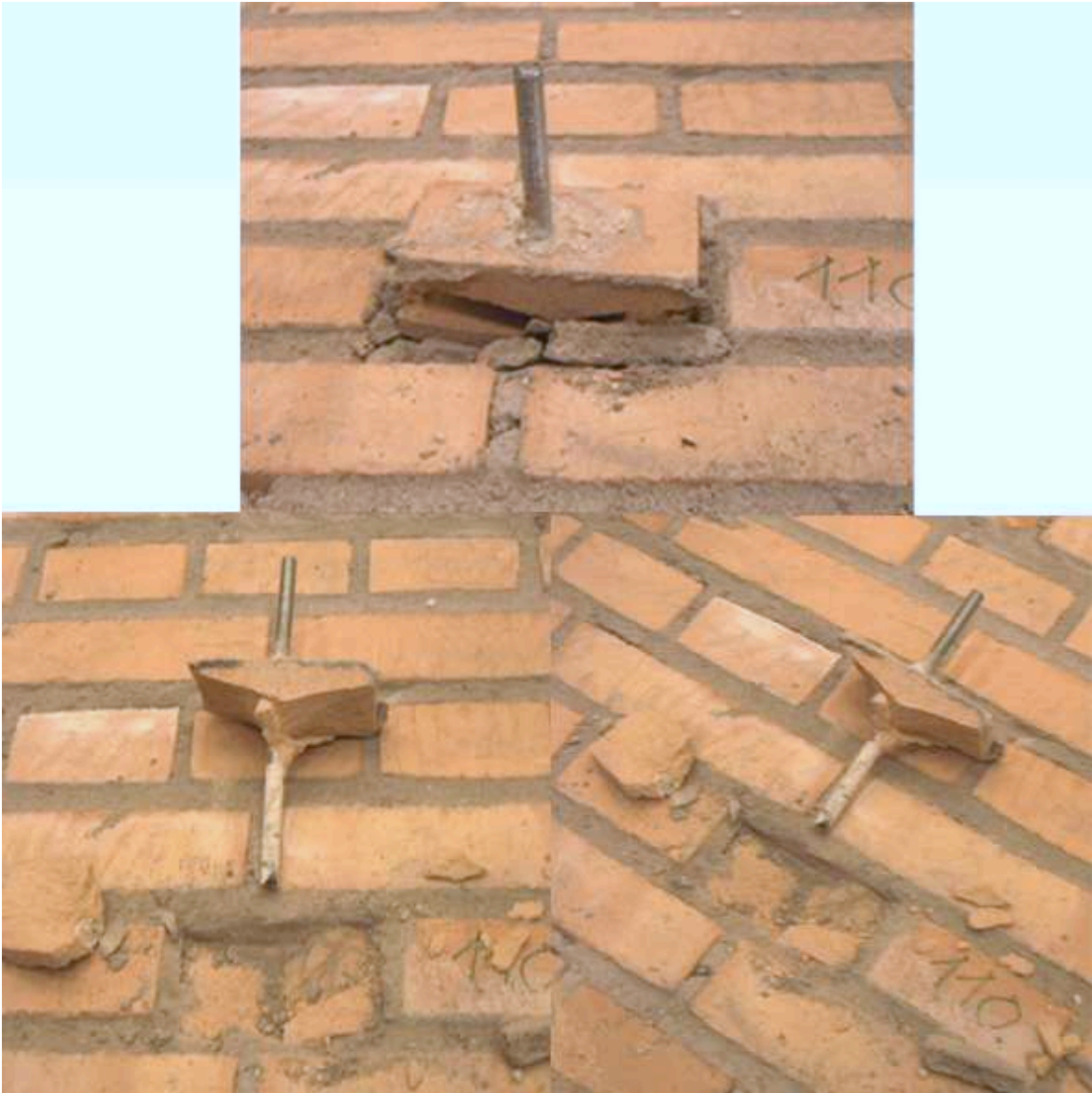
Figure A.55: The failure mode observed
