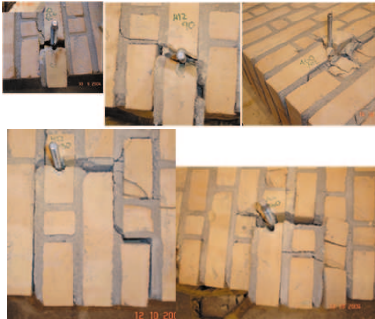
Figure 2.11: Typical splitting failures in masonry
