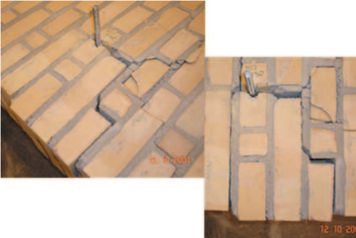
Figure A.131: The failure mode observed
