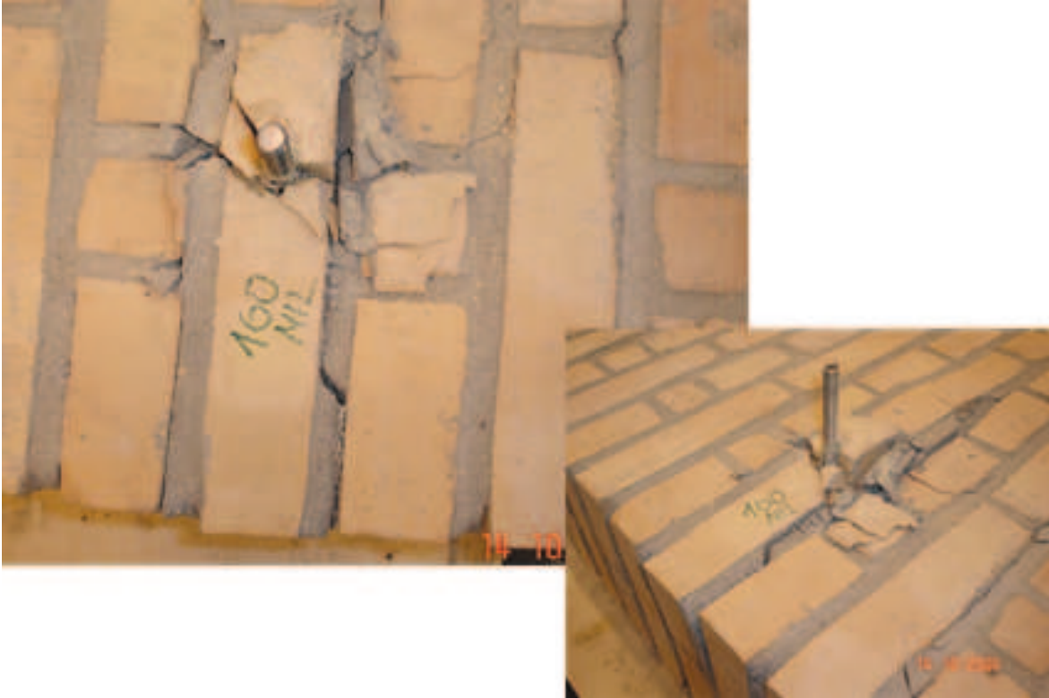
Figure A.129: The failure mode observed
