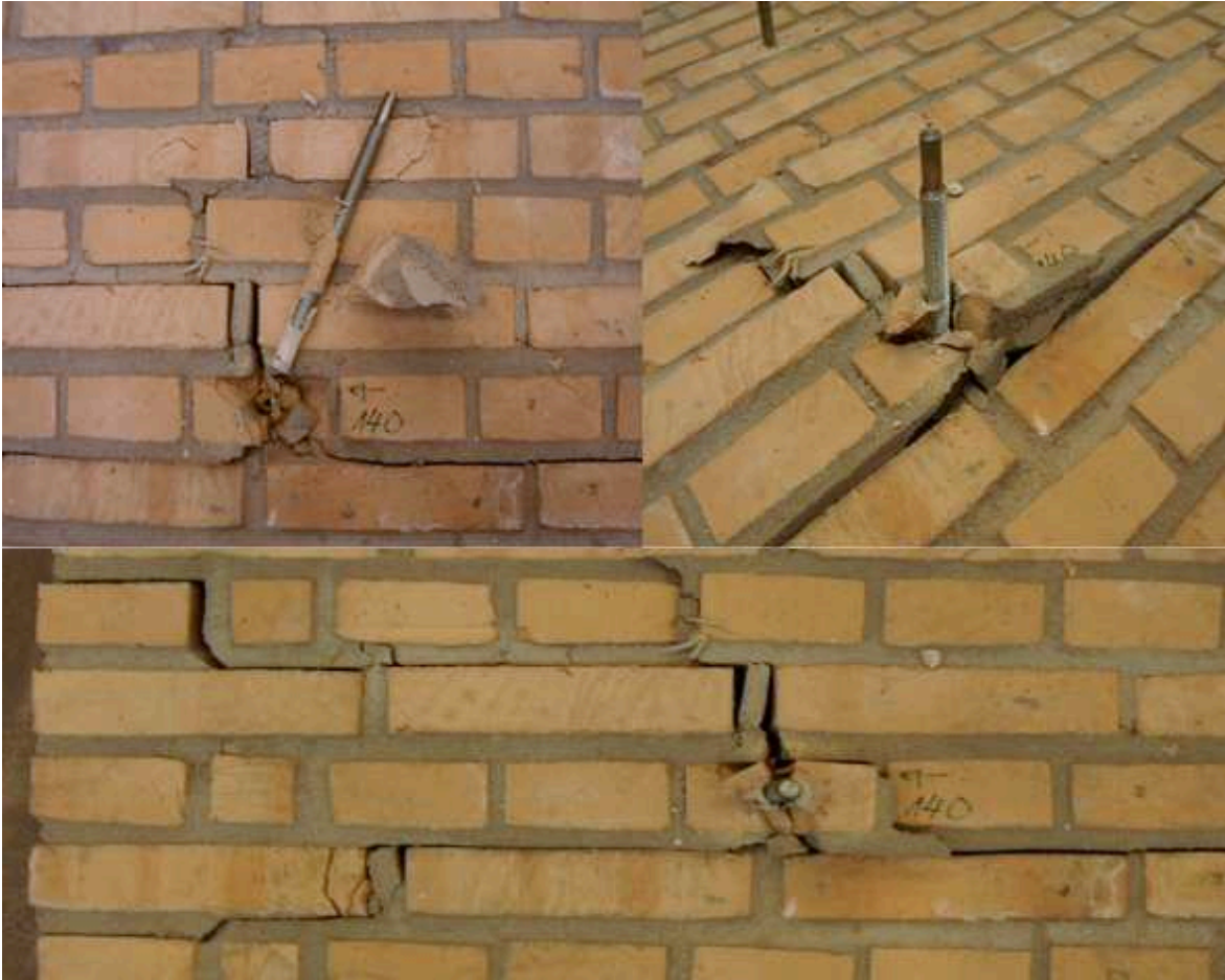
Figure A.81: The failure mode observed
