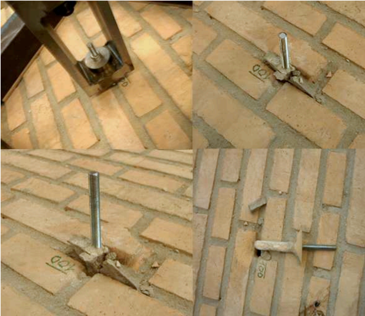
Figure A.85: The failure mode observed
