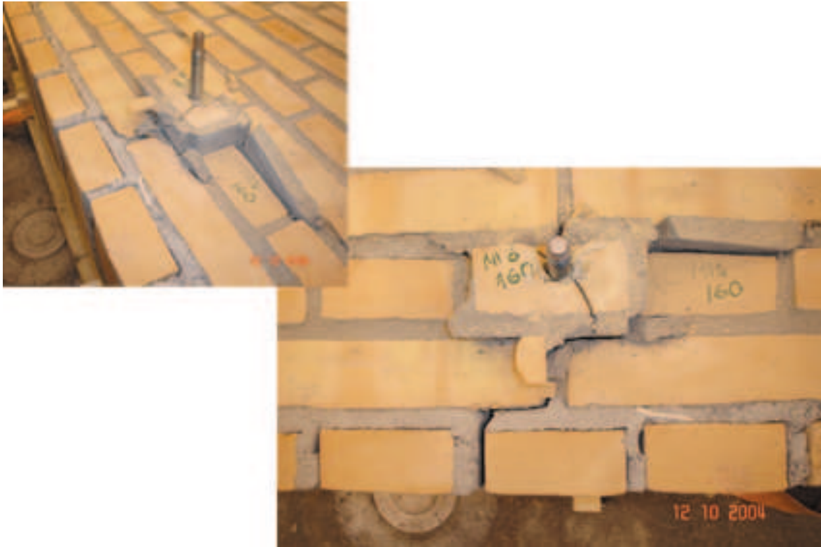
Figure A.147: The failure mode observed
