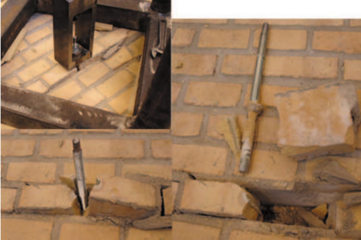
Figure A.11: The failure mode observed
