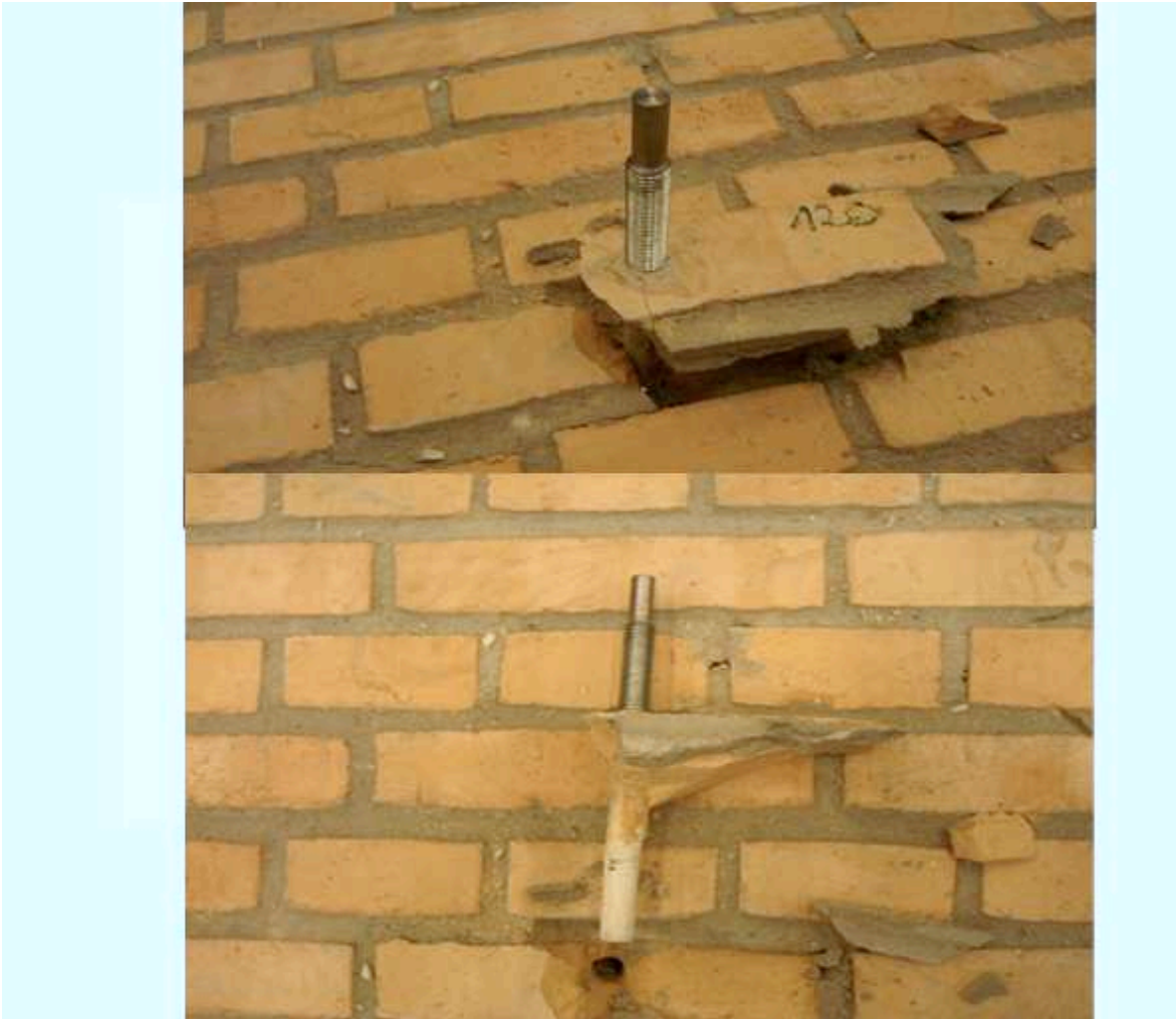
Figure A.33: The failure mode observed
