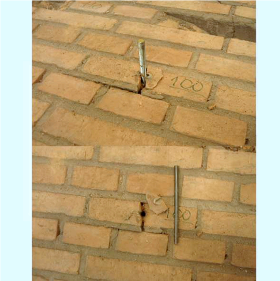
Figure A.15: The failure mode observed
