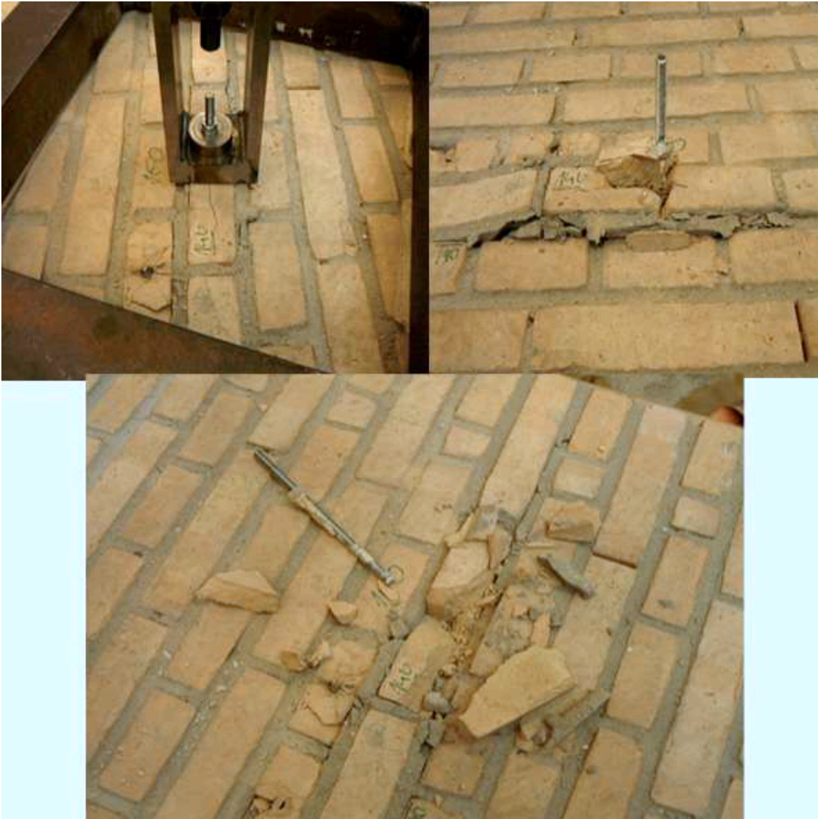
Figure A.19: The failure mode observed
