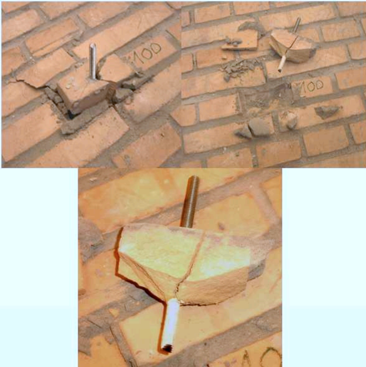
Figure A.53: The failure mode observed
