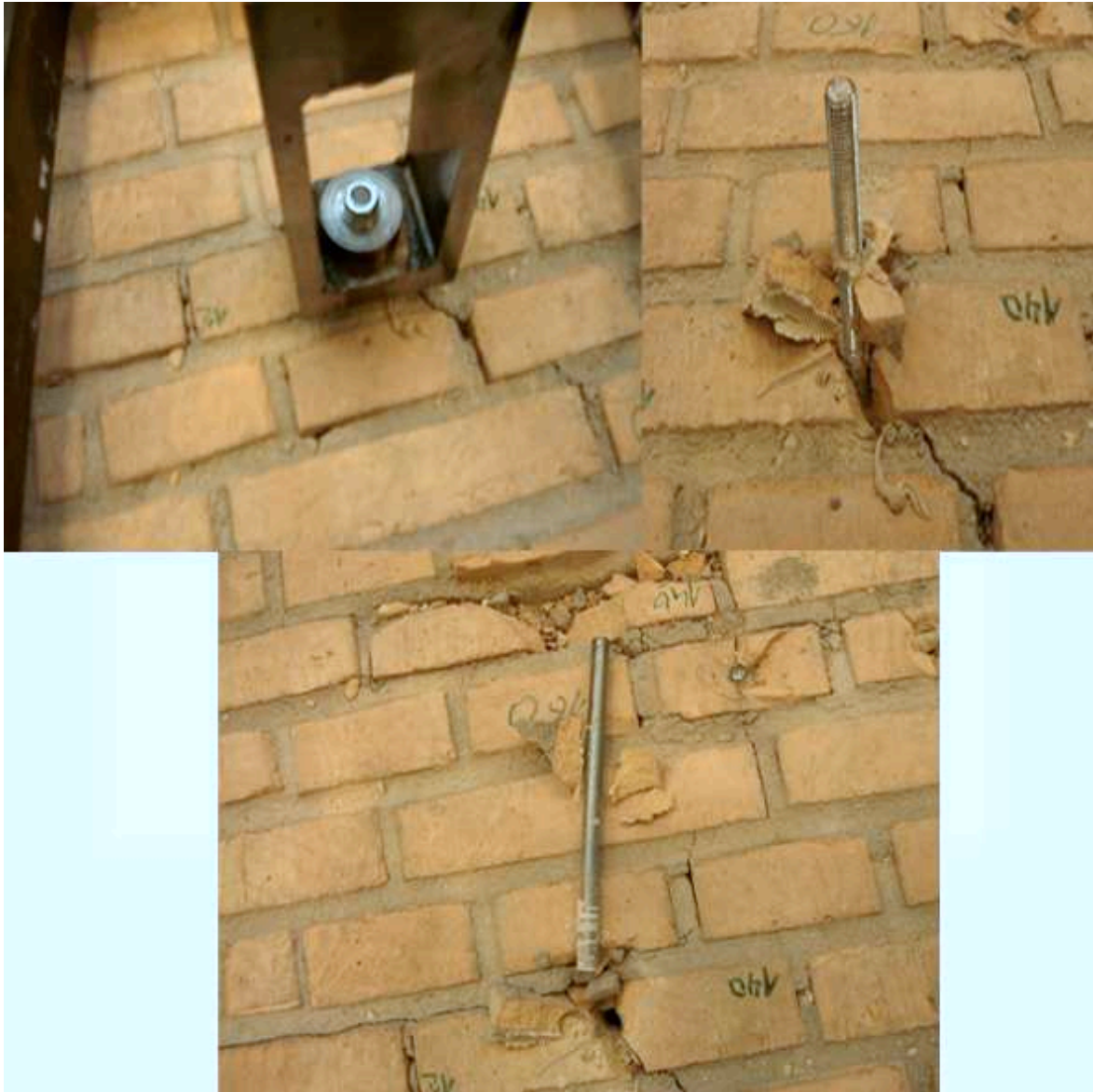
Figure A.27: The failure mode observed
