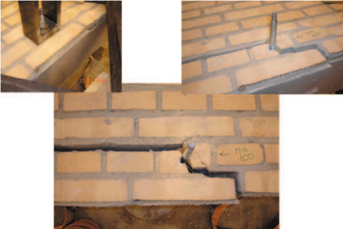
Figure A.145: The failure mode observed
