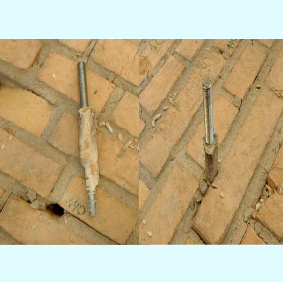
Figure A.97: The failure mode observed
