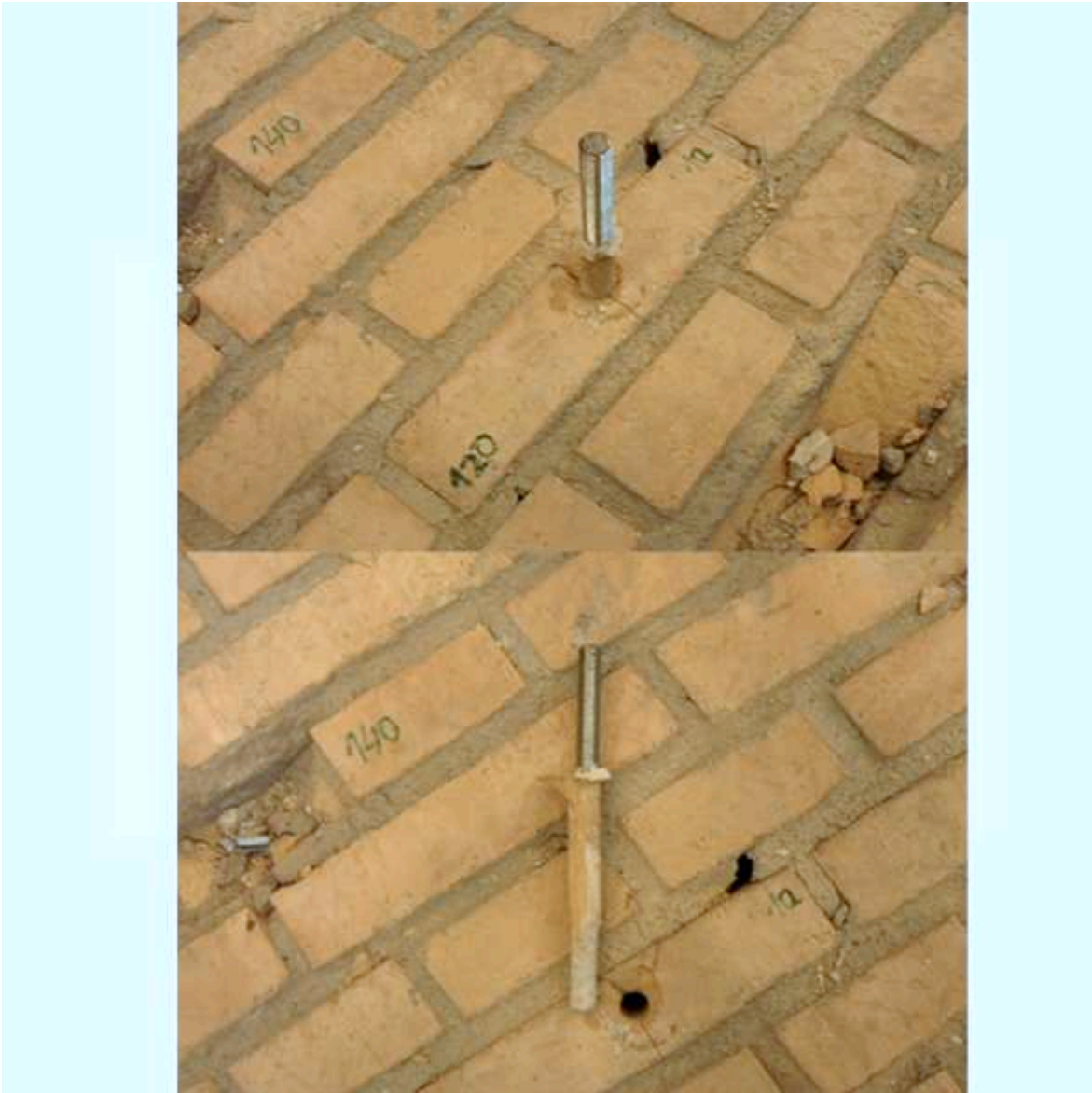
Figure A.25: The failure mode observed
