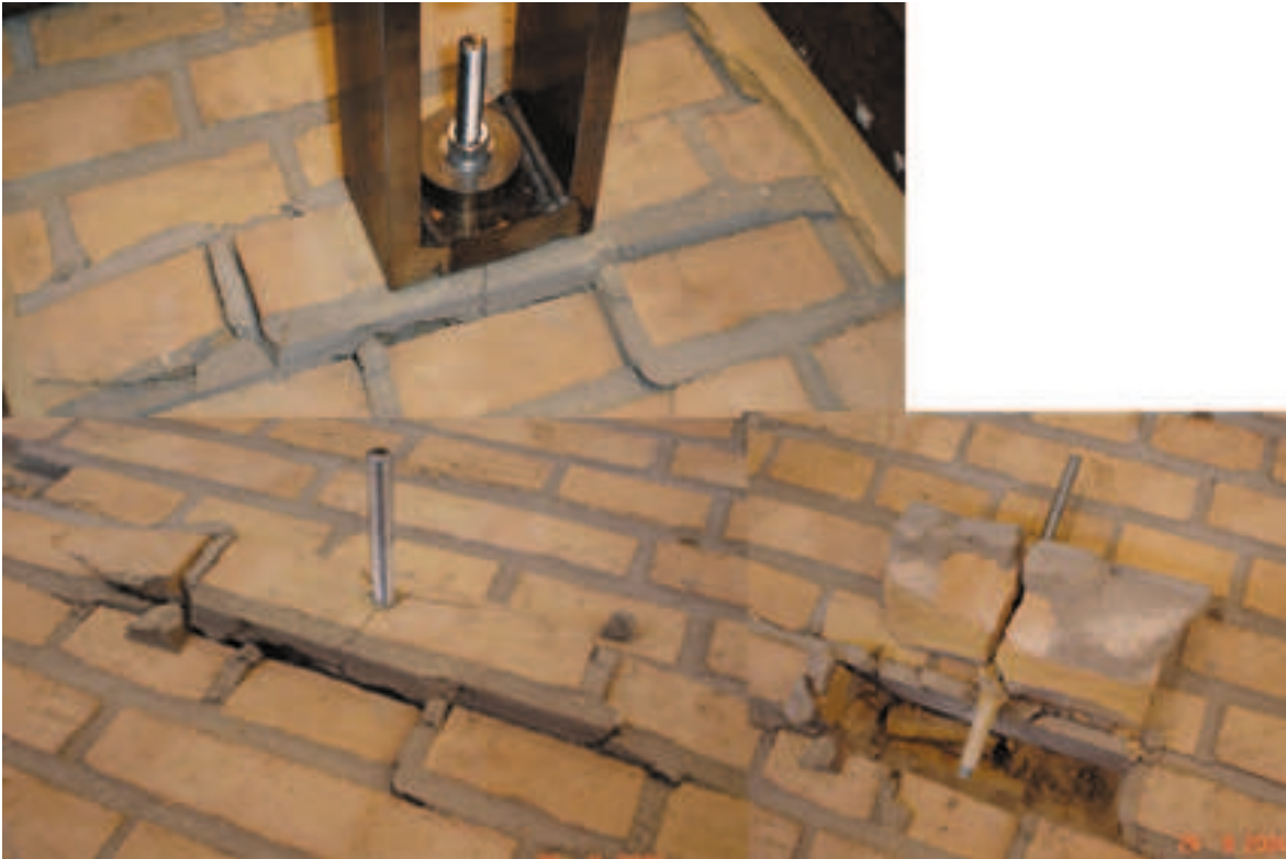
Figure A.7: The failure mode observed
