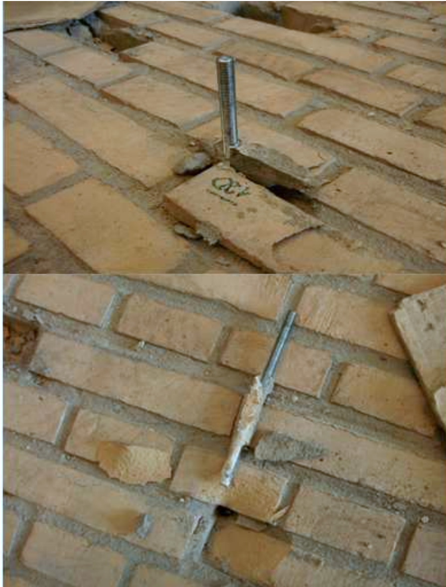
Figure A.87: The failure mode observed
