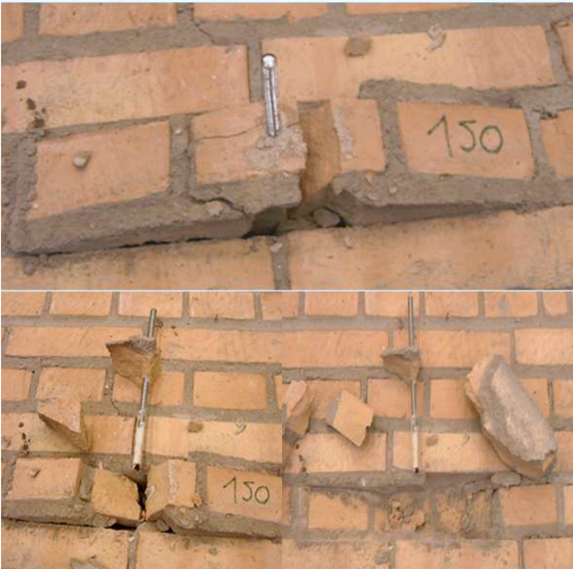
Figure A.63: The failure mode observed
