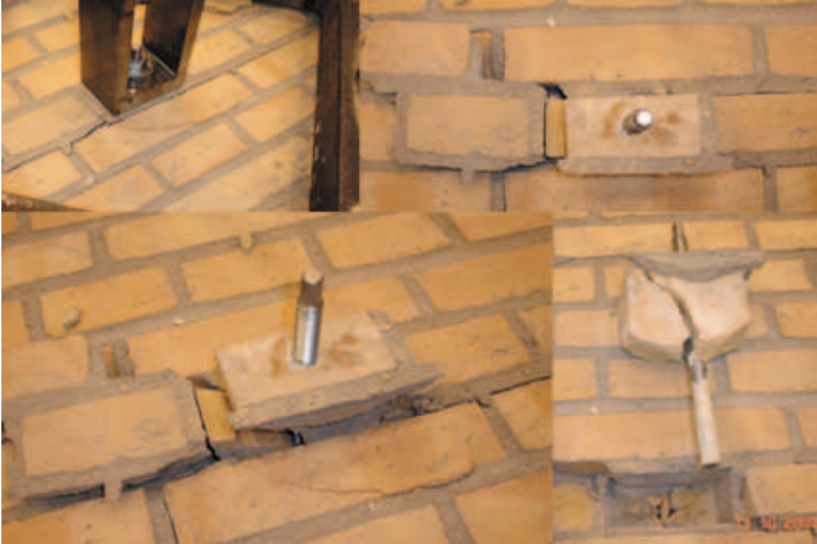
Figure A.47: The failure mode observed
