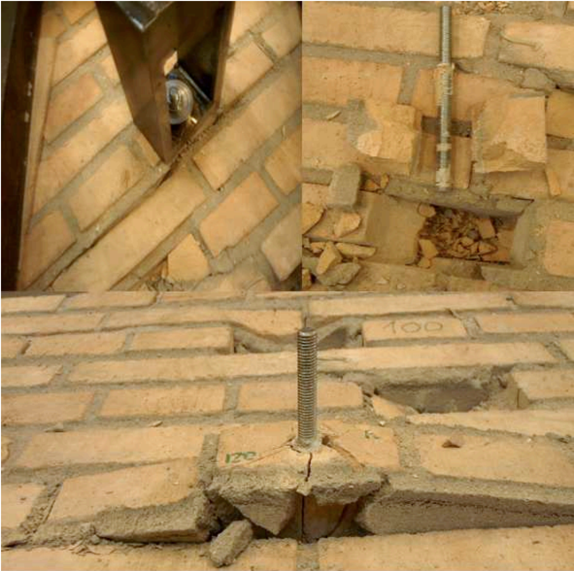
Figure A.71: The failure mode observed
