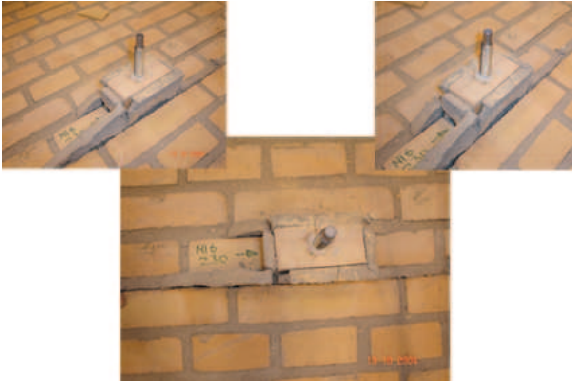
Figure A.149: The failure mode observed
