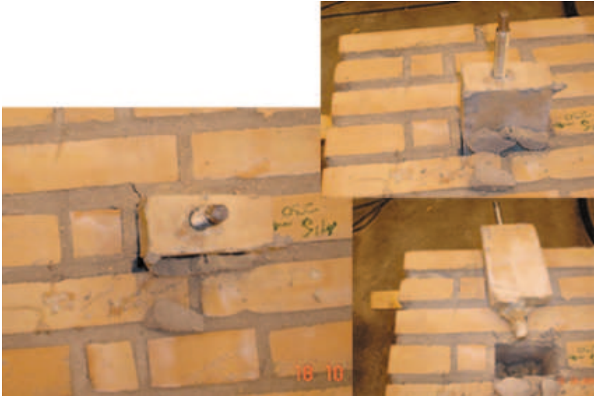
Figure A.125: The failure mode observed
