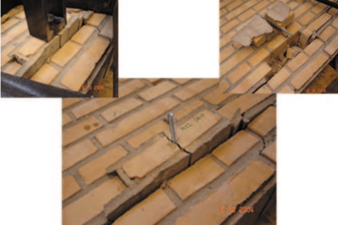
Figure A.141: The failure mode observed
