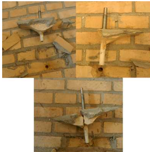
Figure 2.8: Brick-cone failures typically observed in masonry
