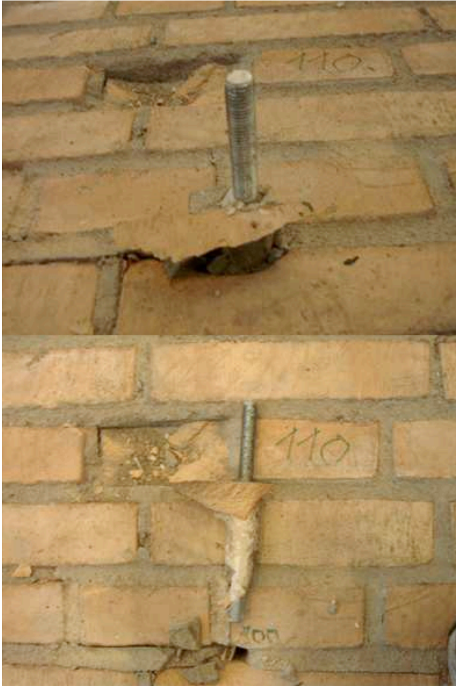
Figure A.93: The failure mode observed
