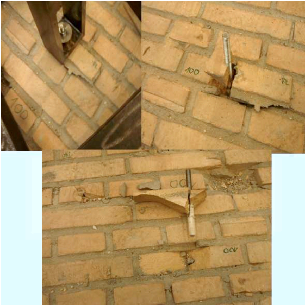
Figure A.23: The failure mode observed
