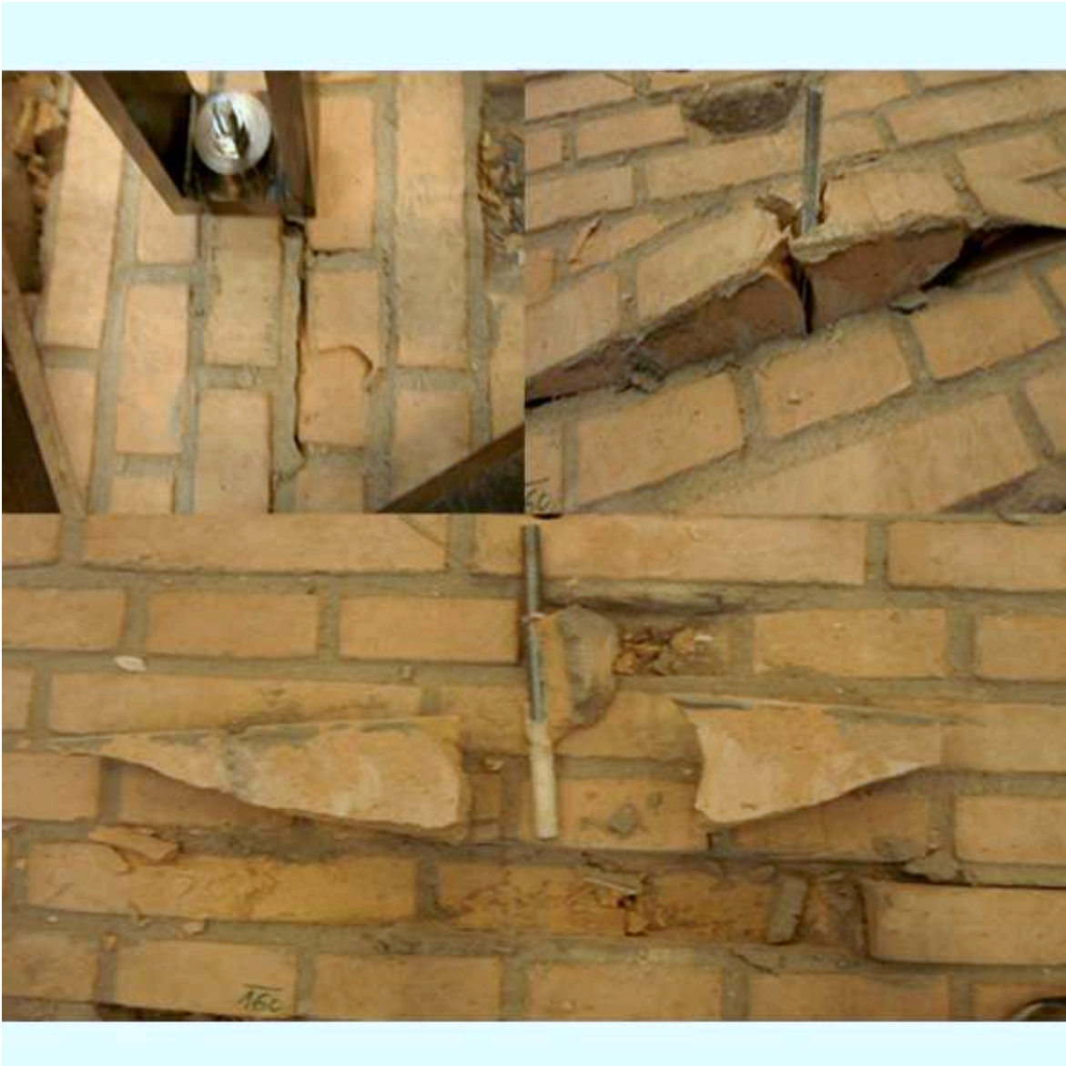
Figure A.29: The failure mode observed
