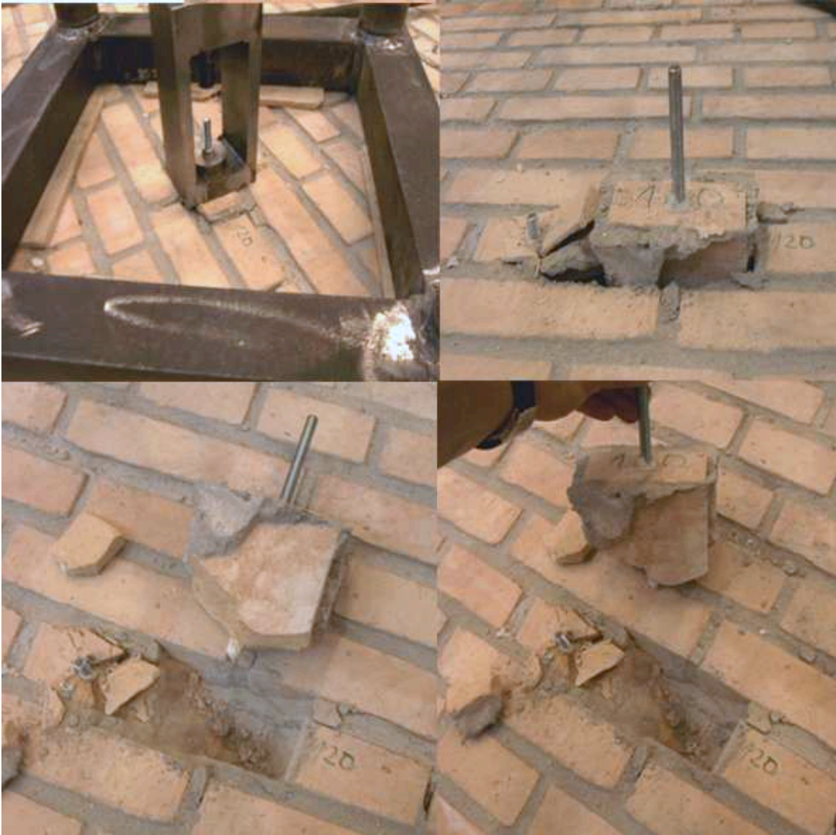
Figure A.57: The failure mode observed
