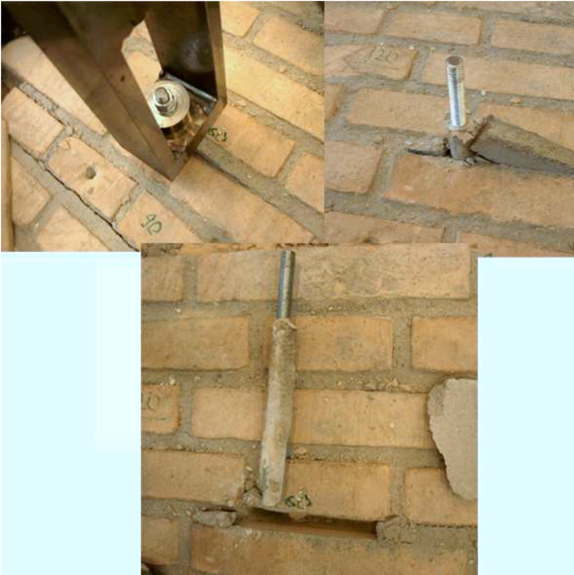
Figure A.99: The failure mode observed
