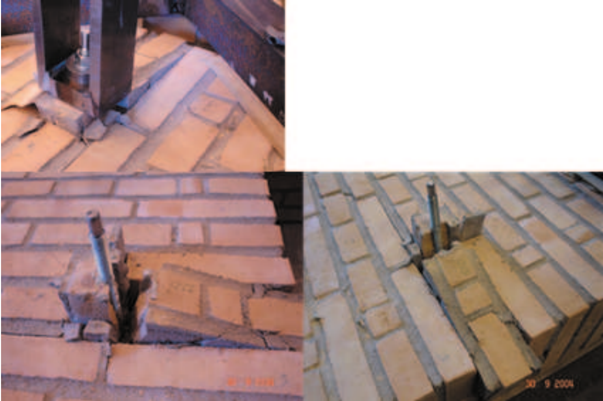
Figure A.137: The failure mode observed
