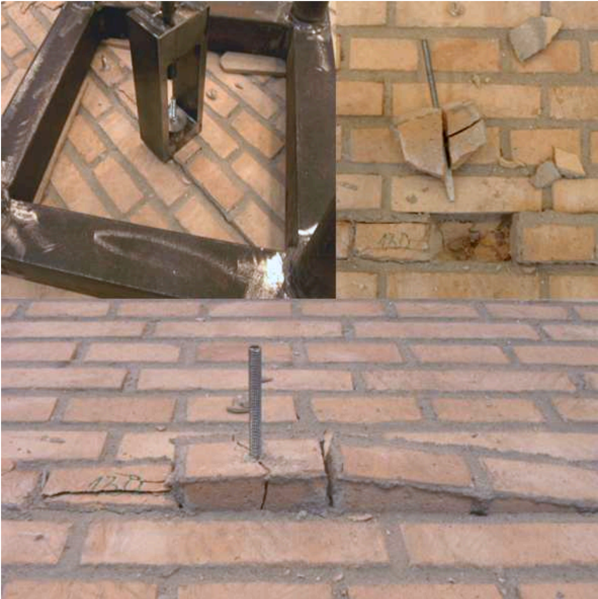
Figure A.59: The failure mode observed
