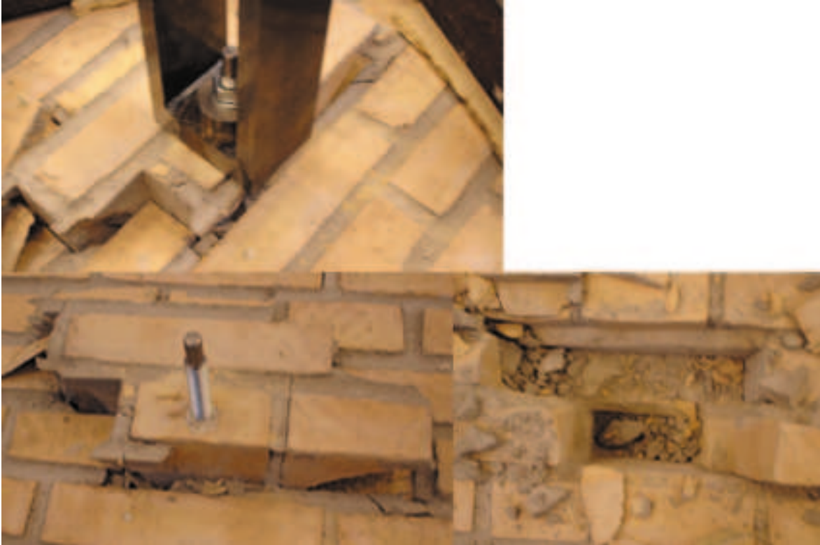
Figure A.45: The failure mode observed
