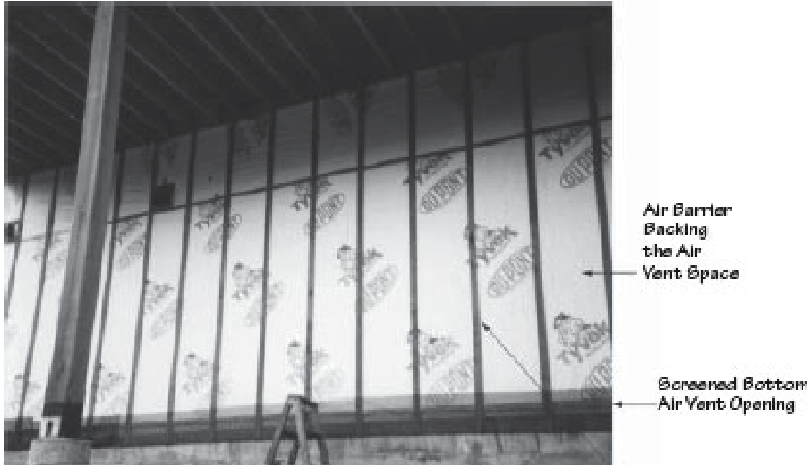
Figure 4: A photo of a ventilated exterior cladding system under construction in Southeast Alaska. (From an English translation of the NBI publication “Byggedetaljer: NBI Byggforsk A542.003”, also published as Alaska Building Research Series HCM-01558, with additions and used with permission, 1988)
