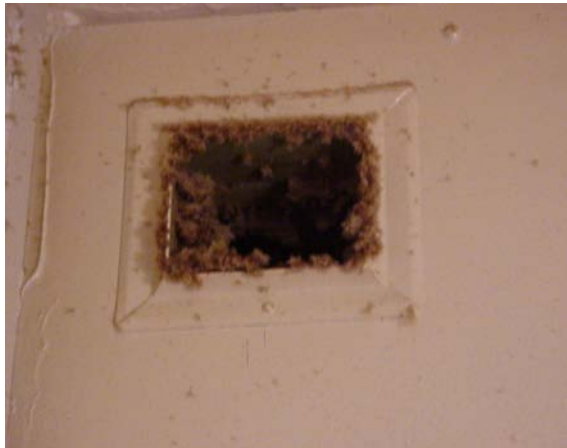
Building element no. 330 Loft ventilations should be established.
