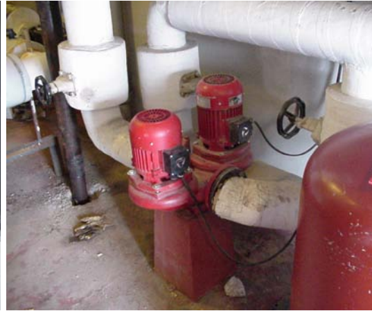
Building element no. 310 Heat pipes are leaking when they are lead through floors. There is poured 100-150 litres on the system every week
