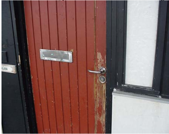
Building element no. 110 Exchange of some doors Building element no. 140 Roof covering is leaking.
