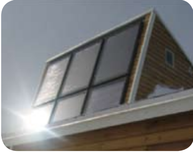
The solar collectors on the low-energy house
