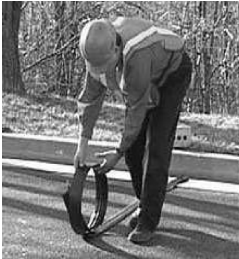
Figure 2.3: The installation of a mobile pneumatic tube traffic detector. The tube is fixed on the highway surface and connected to a registration unit at the roadside [9].
