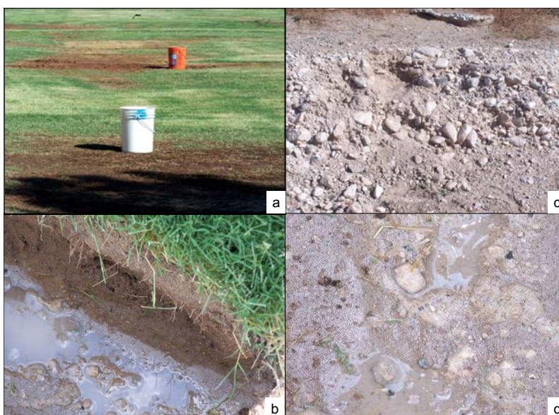
Fig. 5. Salinization of Agustín soil, and the presence of perched water over the flat subgrade at Galatán Park
