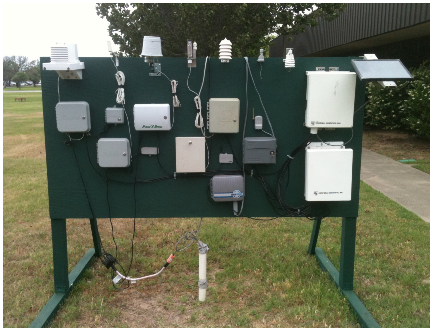
Figure A-4. Outdoor Tested Controllers
