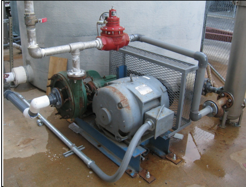
Figure 4.4 : Circulation pump 2 (Capacity - 550 GPM).
