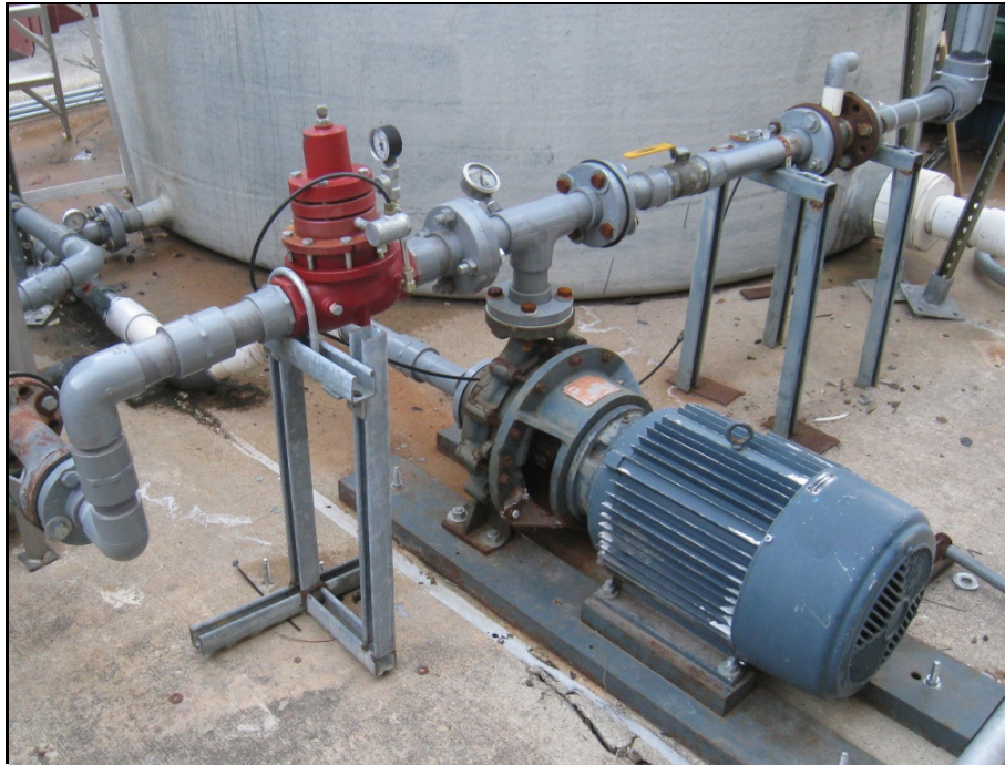
Figure 4.3 : Circulation pump 1 (Capacity - 135 GPM).
