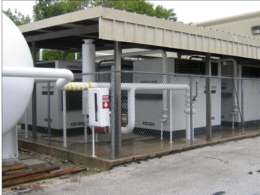
Figure 4.7 : Air compressor network.
