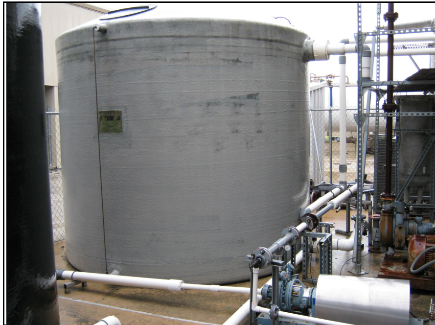
Figure 4.2 : Water supply reservoir.
