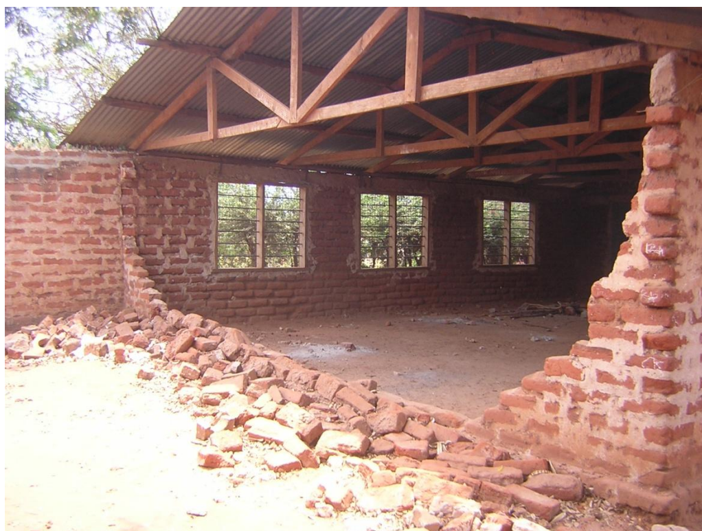
Figure 1 Photograph showing the classroom wall which was destroyed in one of the schools in Chamwino area when parents and guardians protested over their children receiving treatment for urinary schistosomiasis and intestinal worms.
