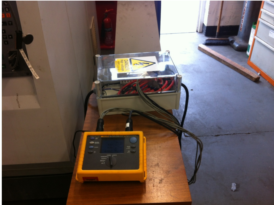
Fig. C.3 Power logger connections
