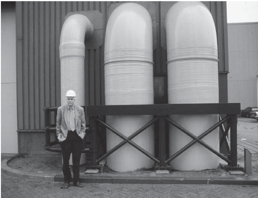
Figure 7 The Roca-III power plant in Rotterdam supplies heating and carbon dioxide to some 120 greenhouses in its vicinity. (Photo by Tim Beatley.)
