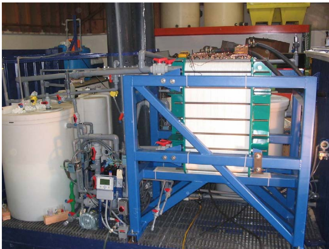
Figure 6. Electrochemical destruction unit for regenerant recycle
