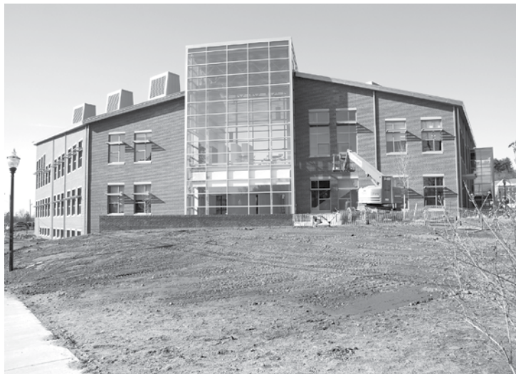
The new Studio Arts Building is almost finished. It is across North Pleasant Street from the Fine Arts Center, to your left in the view.
