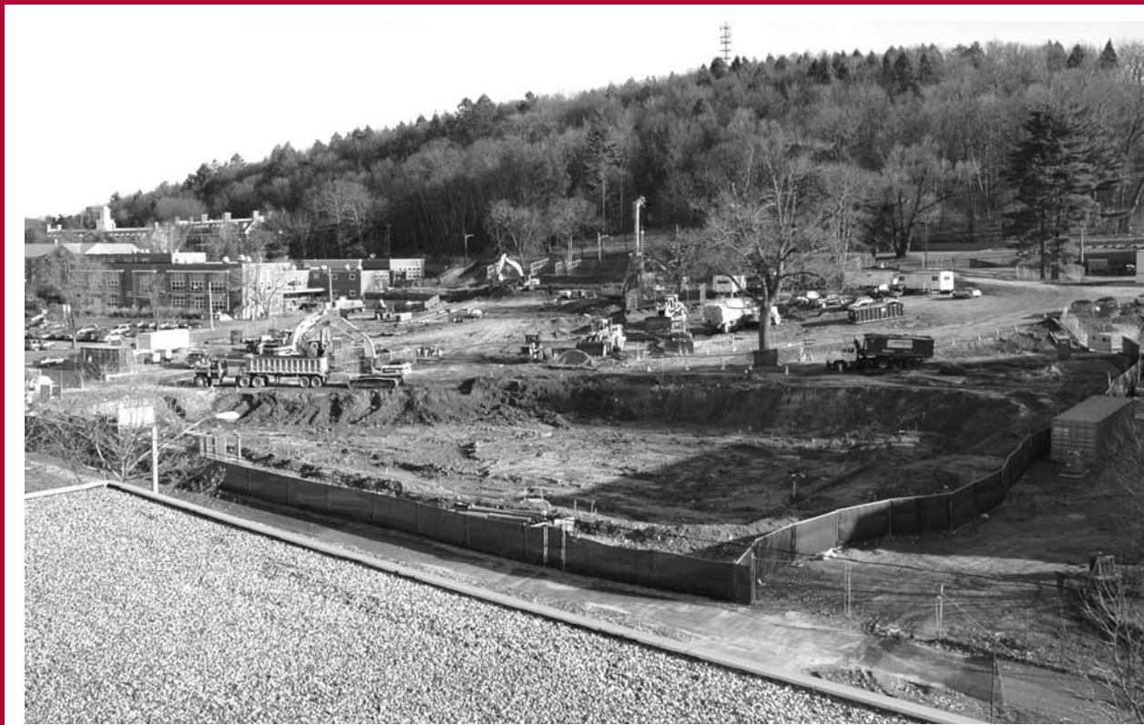
Beginning of construction on what was once Lot 63 parking lot, across N. Pleasant St. from Hasbrouck. At the end of construction sometime in 2008, we will have a new Integrated Science Building.
