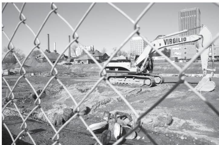
Start of construction on a new student Recreation Center across Commonwealth Avenue from the Mullins Center. This is taken looking east from the Mullins Center, toward Thompson and the Library.
