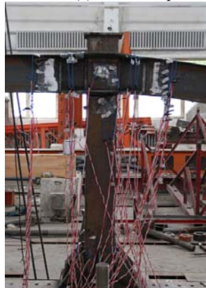
(c) Inclination of column B
