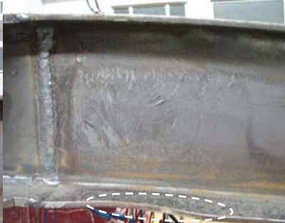
(c) Buckling of beam in joint B
