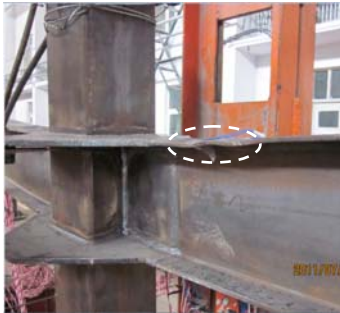
(b) Buckling of beam in joint C
