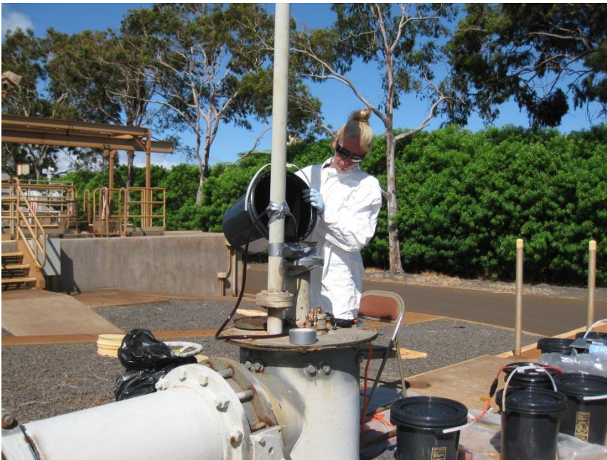
Figure 3-6: Residual dye was poured directly into the well.
