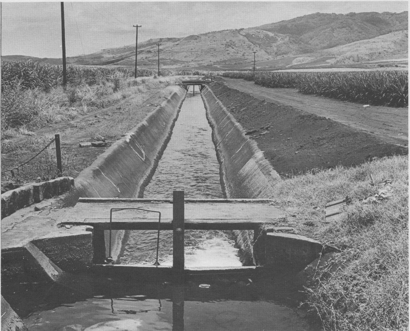
Waiahole Ditch plays a significant role in diverting water from Windward Oahu to the southern slopes of the Waianae range.
